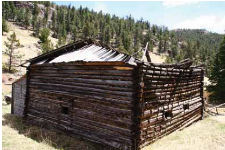
Figure 7: Exterior View of Collapsed Barn
