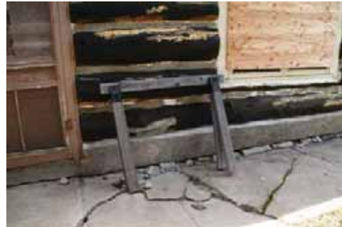
Figure 26: Foundation and Damaged Sidewalk
