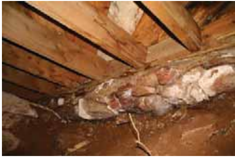
Figure 28: Undercut Foundation in Cellar
