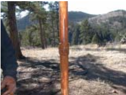
Iron bacterial slime on metal pipe joints.
