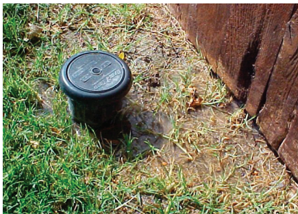
Figure 3: Sprinkler head is too high and leaking.
