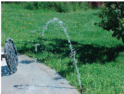
Figure 2: Broken sprinkler head.
