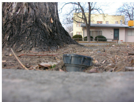
Figure 5: Tilted sprinkler head.
