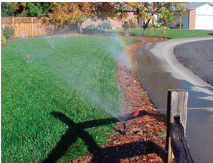
Figure 17: Misting due to excessive pressure.
