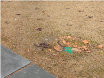
Figure 10: Low valve box.
