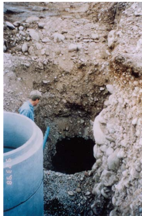
Figure 7. Subsurface void encountered during excavation for utilities in the Roaring Fork Valley. Photo courtesy of Steve Pawlak (HP Geotech).
