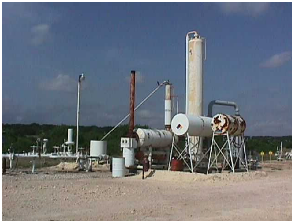
Figure 3-2. Glycol Dehydrator in a Production Field
