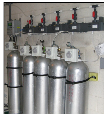
Gas chlorine cylinders. Photo by Serenity Valdez.
