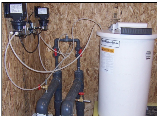
Chlorine injection system. Photo by Paul Kim.
