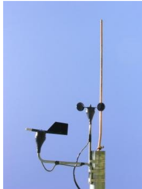
Wind monitoring equipment mounted on tower
