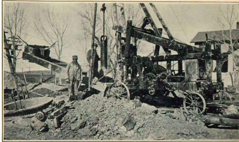
Fig. 16.—Lever-arm method of forcing casing. Ten-inch sand pump on drilling line. At lower left is turntable for soil auger
