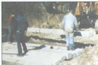
Concrete planks, fastened together and stretched across the streambed, provide an improved ford crossings.
