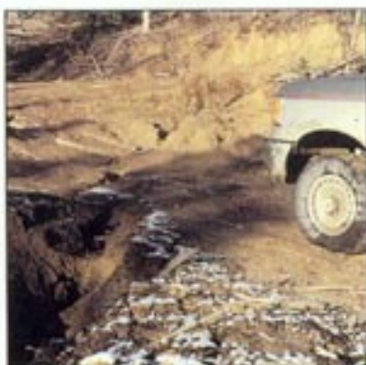
Before grading, it may be necessary to loosen hardened or deep rutted road surfaces. Ripper shanks on a road grader are effective. Road repairs should occur before the wet season. Special attention is needed on steep slopes or curves where greater road surface wear occurs.
