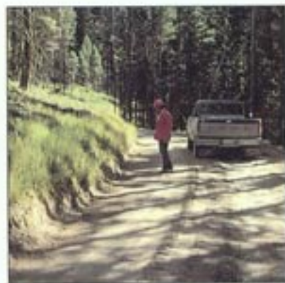
Grader damage to inside ditch toe slopes exposes an easily erodible surface and is a source of sediment. Slow, controlled grading is often the solution, and it can also avoid damage to ditches, culverts, and cutbanks.
