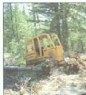
Road restoration includes pulling up roadside berms to prevent channeling water, ripping compacted areas, restoring natural drainage, and reseeding with appropriate grasses.
