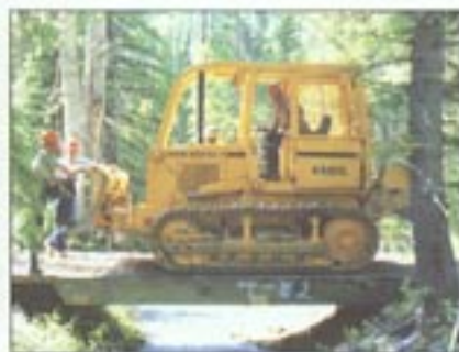
Along with its portability, this temporary bridge is strong enough for all harvesting activities.
