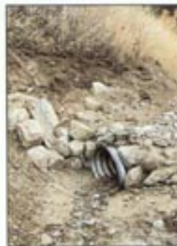
Drop inlets (left photo) installed at the head of a ditch relief culvert slow the flow of water, help settle-out sediment, and protect the culvert from plugging. Rock armored inlets (right photo) prevent water from eroding and undercutting the culvert and flowing under the road.
