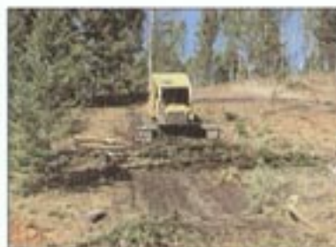
Machine-made ruts on hillside soils can easily become channels for surface water erosion.
