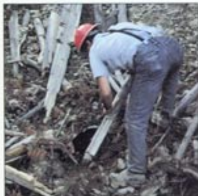
Hand, shovel, and chainsaw work are usually all that culvert maintenance requires. But don't delay! Delay in cleaning a blocked culvert or ditch can result in a damaged road which requires costly reconstruction.
