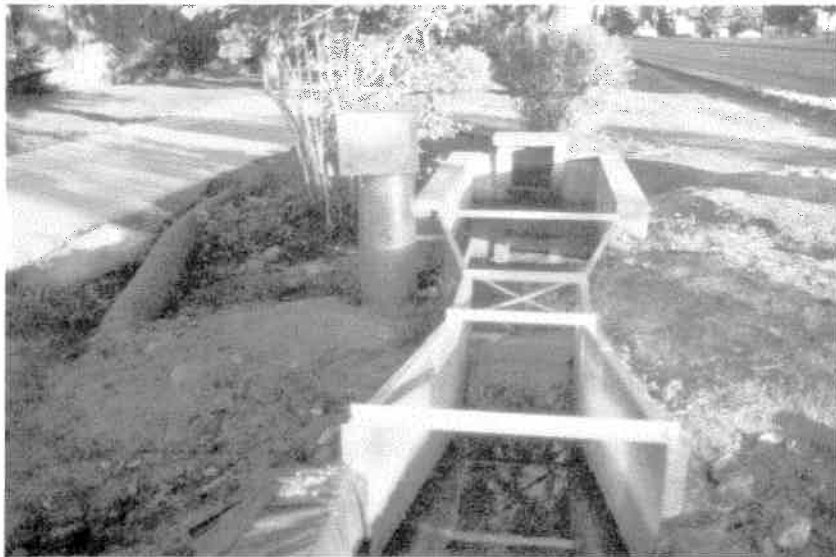
Parshall flume on University of Colorado campus
