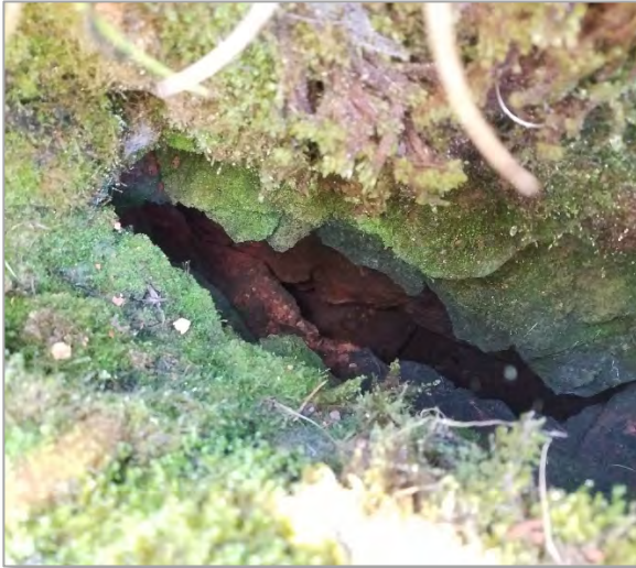
Figure 4-75 – Venting Fracture w/ Moss
