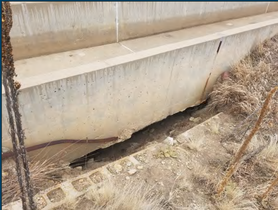
Subsidence under aqueduct
