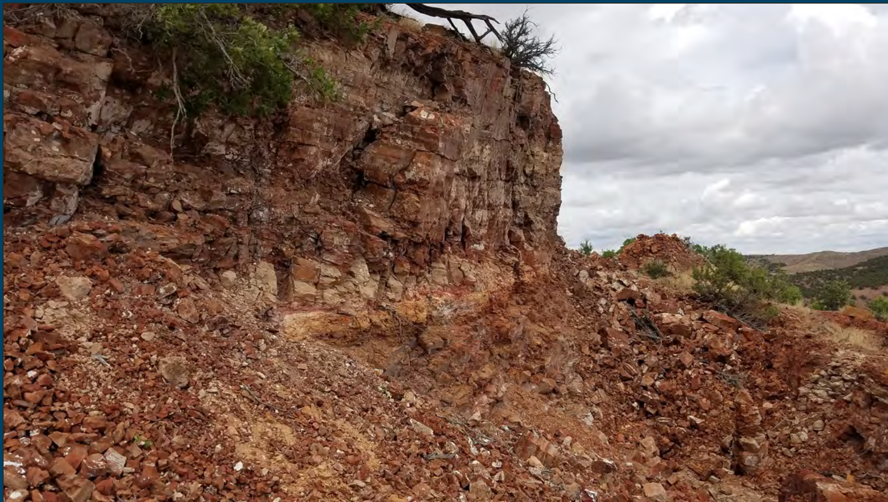
Large fracture looking North
