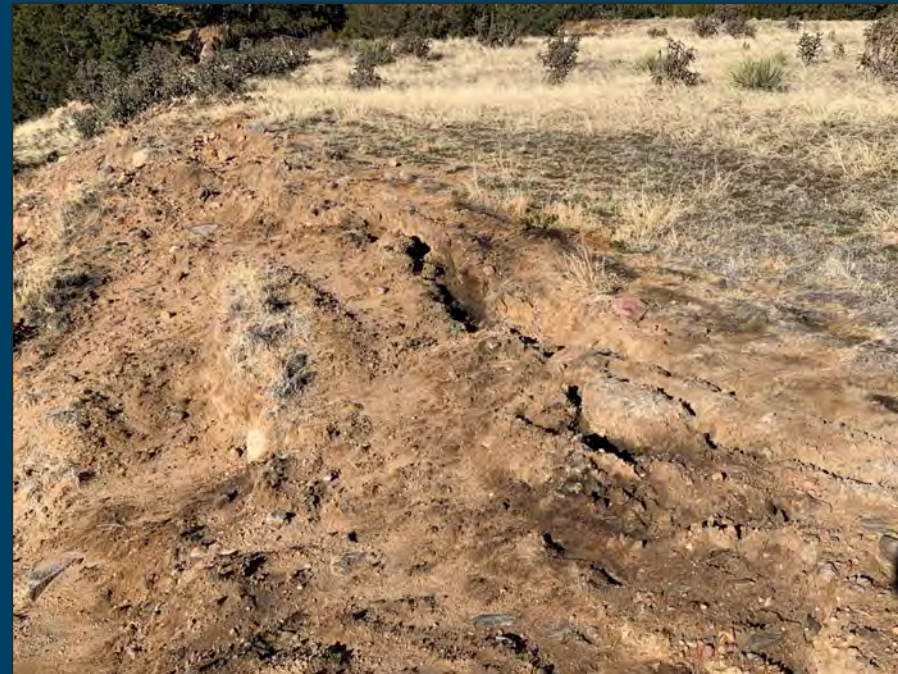
Slumping near vents
