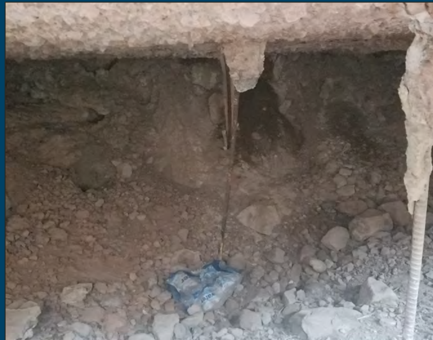
Subsidence under aqueduct
