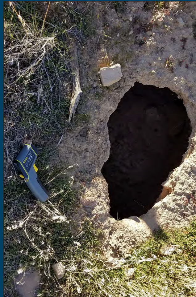
Small subsidence on upper fracture
