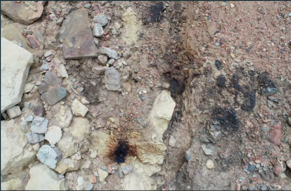
Western vents with creosote staining
