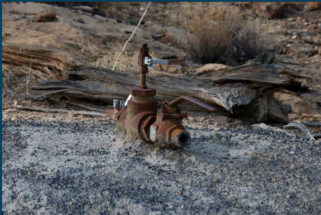
Open wellhead venting H 2 S gas
