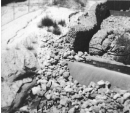
PHOTO 10.5-1—Failed spillway gabion wall
