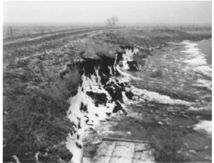
PHOTO 6.2—EROSION OF UPSTREAM FACE DUE TO LACK OF PROTECTION AGAINST WAVE ACTION.
