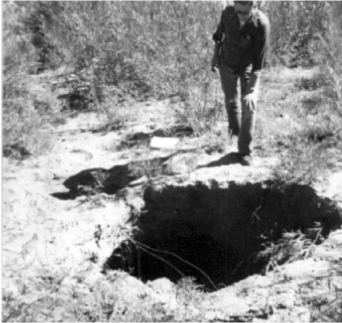
PHOTO 9.4-1—SINKHOLE ON DOWNSTREAM SLOPE ABOVE OUTLET CONDUIT. Failure occurred as described in Figure 9.4-3.
