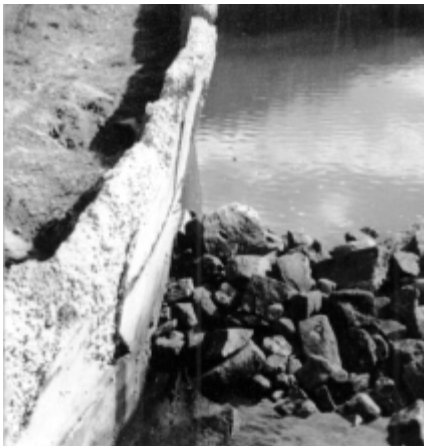
PHOTO 10.5-1—Deterioration of right D/S wingwall of spillway.
