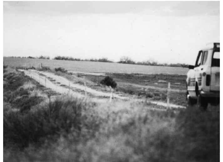
PHOTO 7.5-2—LOW AREA IN THE CREST OF A DAM, caused by a foundation failure.
