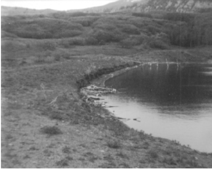
PHOTO 6.5-7—EROSION AT UPSTREAM FACE
