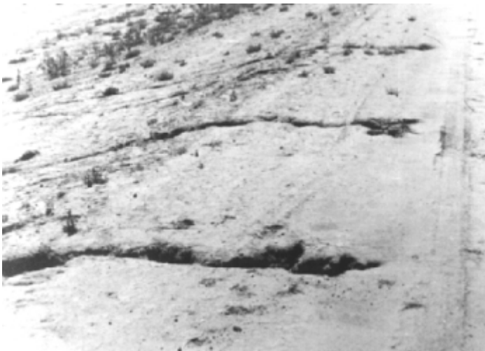
PHOTO 7.5-6—RUNOFF GULLIES FORMING ON THE DOWN-STREAM SHOULDER OF THE CREST
