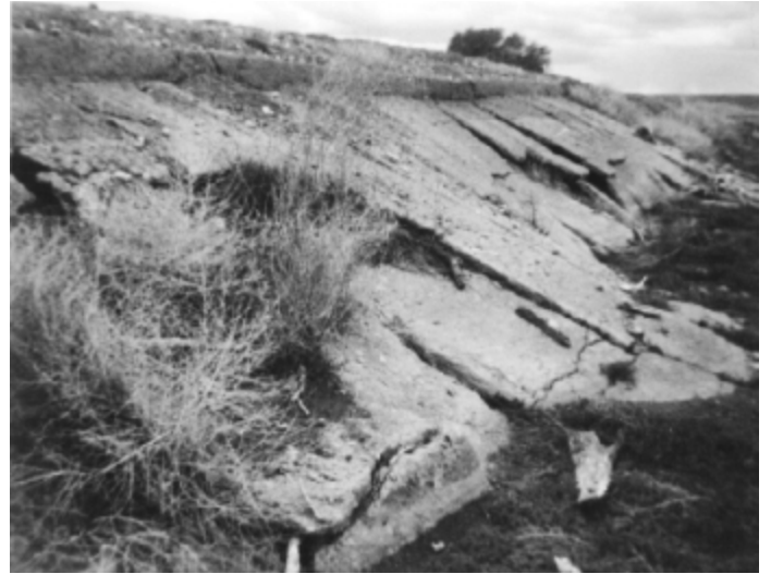
PHOTO 6.5-5—BADLY DETERIORATED CONCRETE FACE
