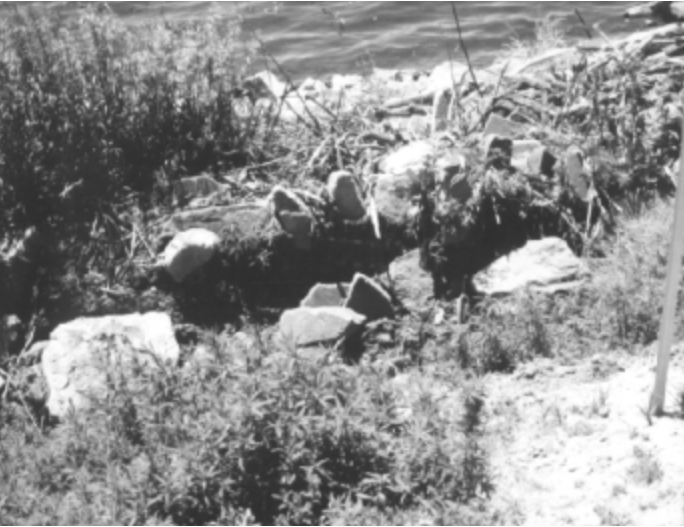
PHOTO 6.5-2—CRACK IN UPSTREAM SLOPE
