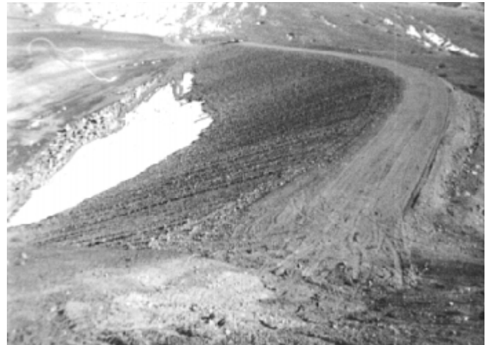
PHOTO 7.5-9—CAMBER INCORPORATED INTO CREST DURING CONSTRUCTION. Camber is greatest over highest section of the dam
