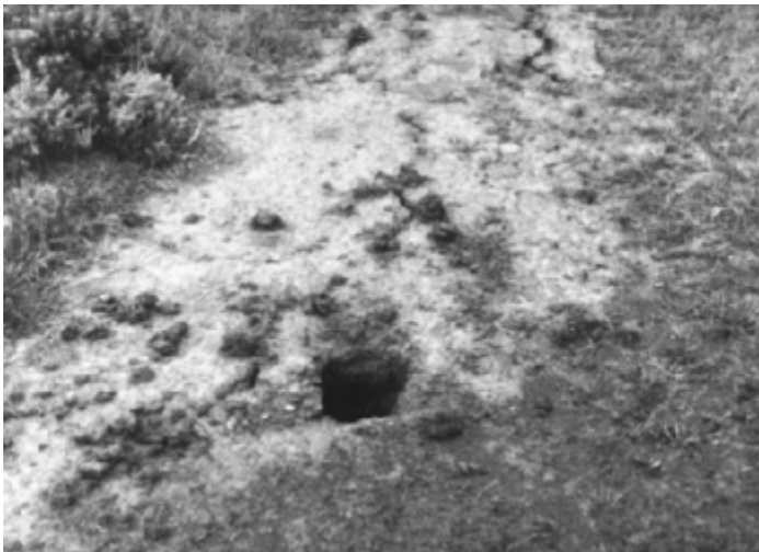
PHOTO 7.5-5—RODENT HOLE FOUND ON THE CREST OF A DAM
