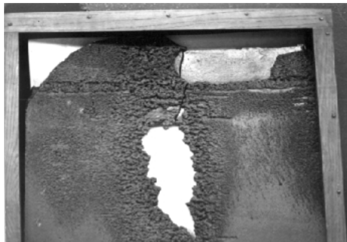
PHOTO 9.3-2—CAVITATION DAMAGE TO STEEL PIPE LINER. Cavitation has eaten through steel to expose concrete behind liner.
