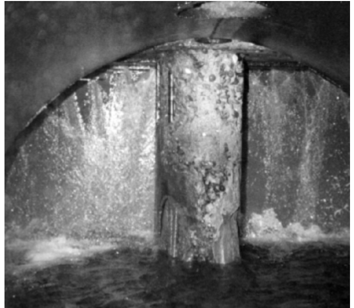
PHOTO 9.8-3—SIDE BY SIDE SLIDE GATES Gate leakage and cavitation damage to bull nose pier. Note exposed reinforcing steel. Air vent pipe at top of photo.
