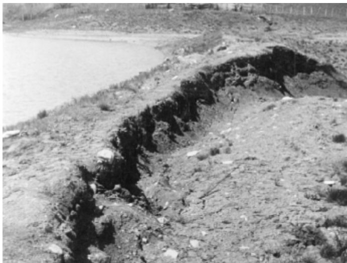
PHOTO 7.5-1.B—VERTICAL DISPLACEMENT ON THE CREST OF A DAM. This vertical movement was associated with a slip on the downstream face.
