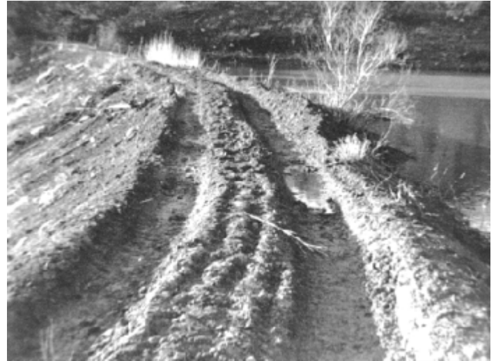
PHOTO 7.5-7—RUTS IN THE CREST OF A DAM
