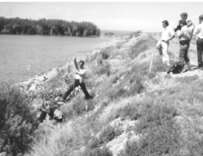
PHOTO 6.5-3—CRACK IN UPSTREAM SLOPE
