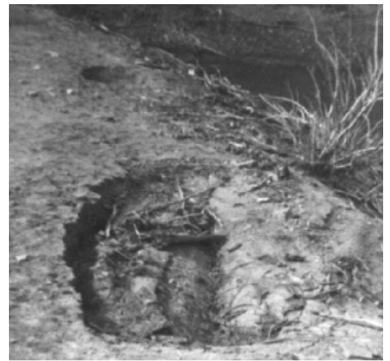
PHOTO 7.5-3—SINKHOLES IN THE CREST OF A DAM, caused by consolidation of low density embankment material.
