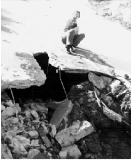
PHOTO 10.5-4—FAILED SPILLWAY Fracturing of spillway chute slab
