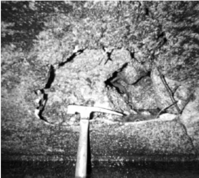
PHOTO 9.8-1—OUTLET—INTERNAL EROSION Hole in cast-in-place concrete lining, caused by turbulence and erosion.
