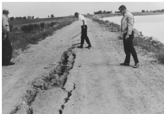
PHOTO 7.3-1—SEVERE LONGITUDINAL CRACKING. Cracking pattern indicates horizontal movement between adjacent sections of the dam. Note the close parallel cracks.
