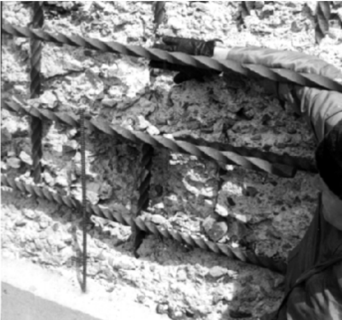
Photo 11.4-3—Structural damage. Spalling has exposed reinforcing.
