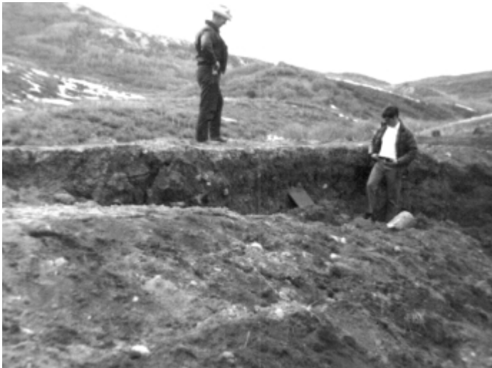
PHOTO 7.5-1.A—VERTICAL DISPLACEMENT ON CREST.
