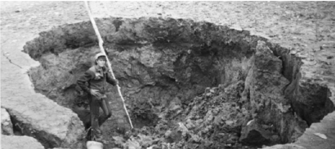
PHOTO 6.5-8—21'X21' SINK HOLE IN RESERVOIR BASIN
