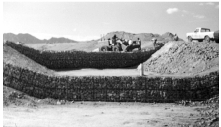
PHOTO 10.4-1—GABION DROP STRUCTURE. A special type of rock protection against erosion.
