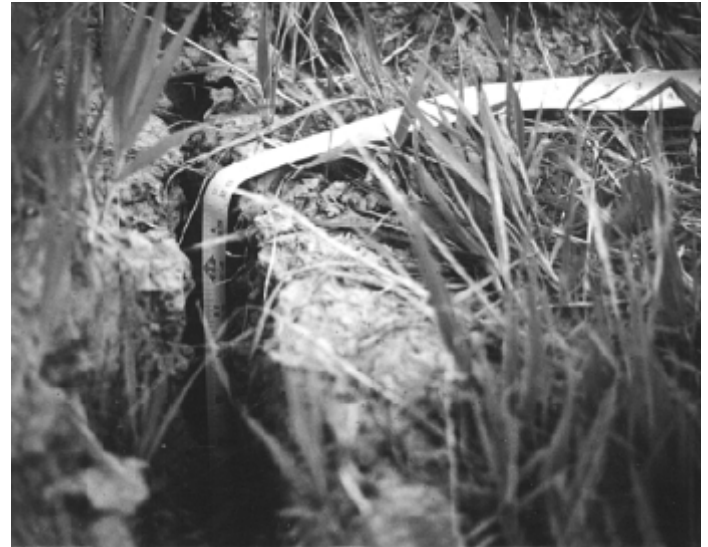
PHOTO 8.3-1—Three-fourth-inch-wide crack, well hidden in grass cover.
