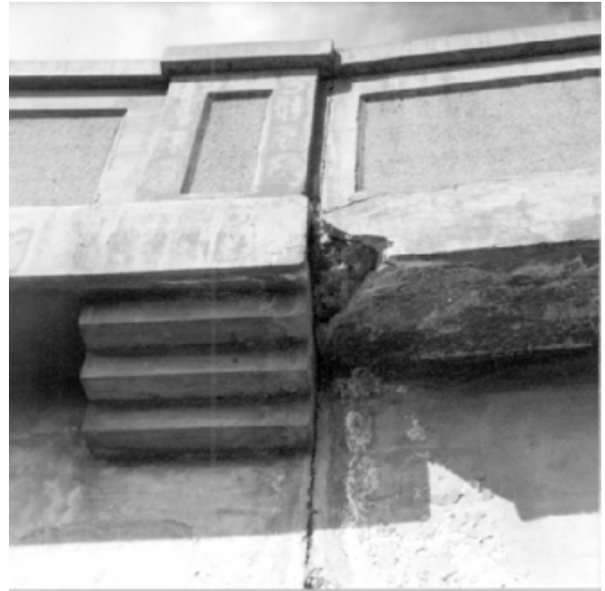
PHOTO 11.4-1 CRACK AT VERTICAL CONSTRUCTION JOINT. Note evidence of minor leakage and spalling adjacent to joint.
