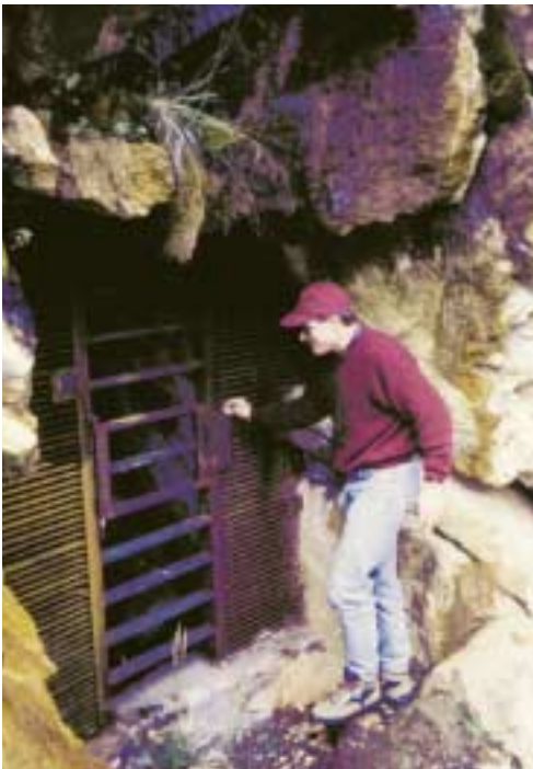
A STEEL GRATE BARRIER AT AN ADIT WITH BARS ALLOWING BAT ACCESS AND A LOCKING DOOR
