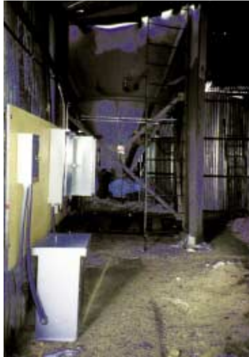
FULL-SCALE LIMESTONE INJECTION SYSTEM WITH LIMESTONE HOPPER, FEEDER SYSTEM AND CONTROL PANELS
