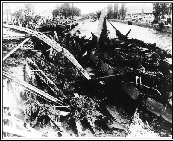
Bridges across Cherry Creek on Colorado Boulevard, Stout and Champa Streets were completely destroyed. Partial damage was done to the Logan Street Bridge. Photo courtesy of Denver Public Library.
