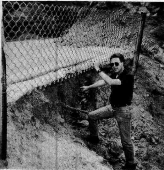
Wash Out Damage - Will Rogers Shrine Road above Cheyenne Mtn
