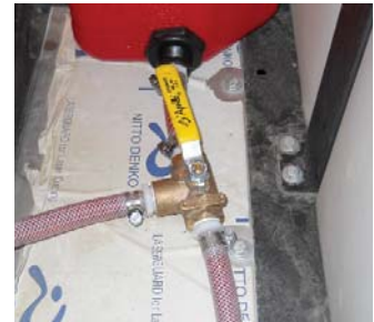
Valve position for water
