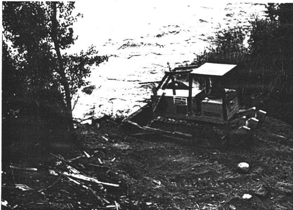
A rock jetty was constructed during the flood to lessen erosion on June 24, 1983.
