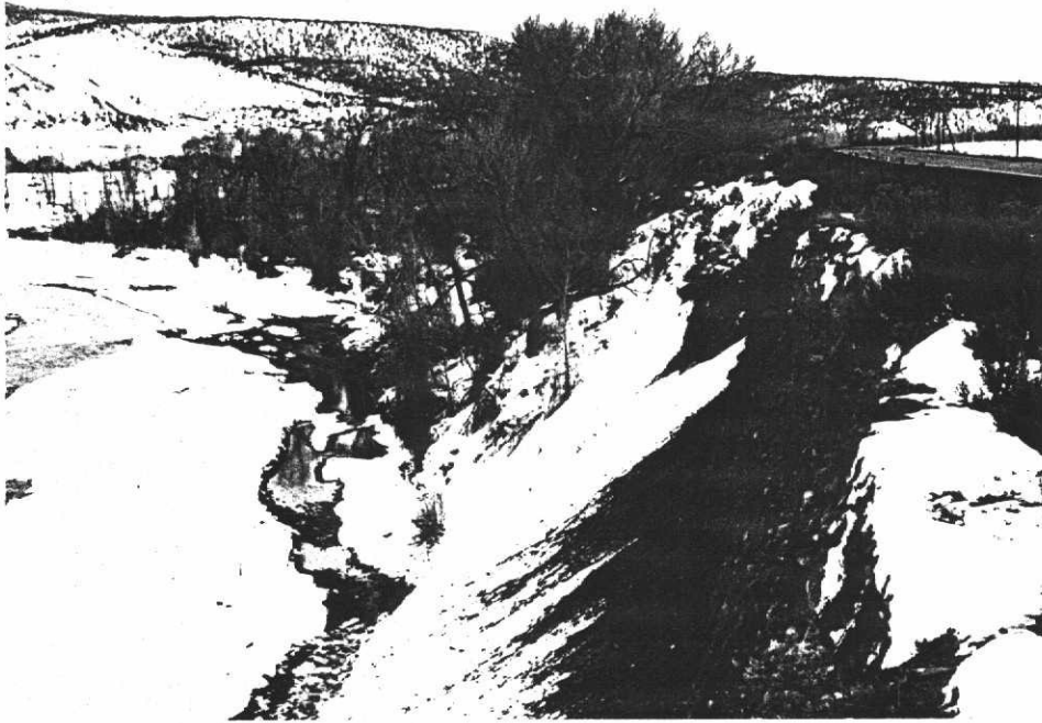
Left bank severely eroded adjacent to Colorado Highway 550.
