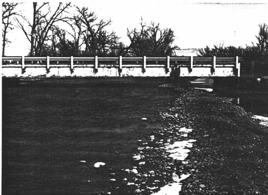
Upstream of Blossom Road. Sediment build-up 6 feet deep.
