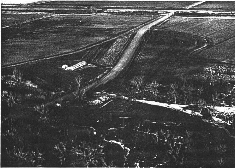
Upstream of County Road B - Erosion of road-way embankment. Riprapping needed.
