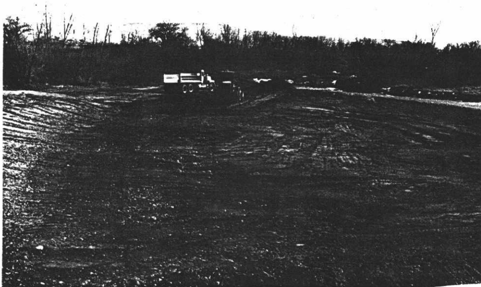
Upstream of County Road 1700 - A large sand bar that needs to be removed because the river is eroding roadway abutment.
