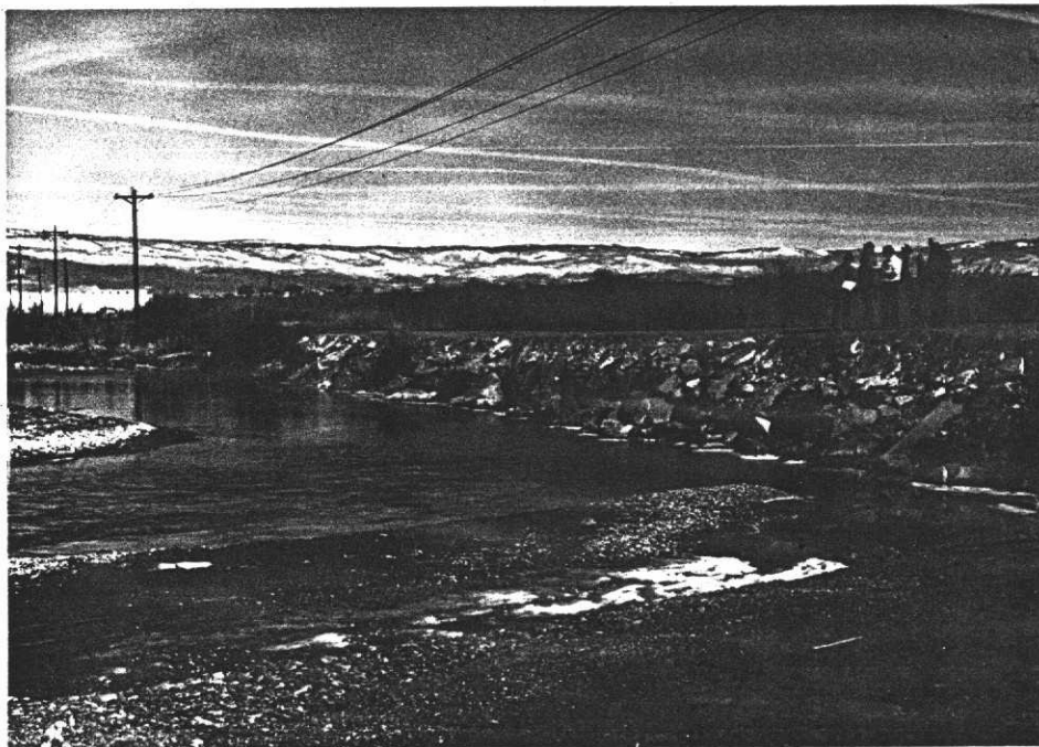
Road repair to County Road 1600 - A cease and desist order was issued by Corps.
