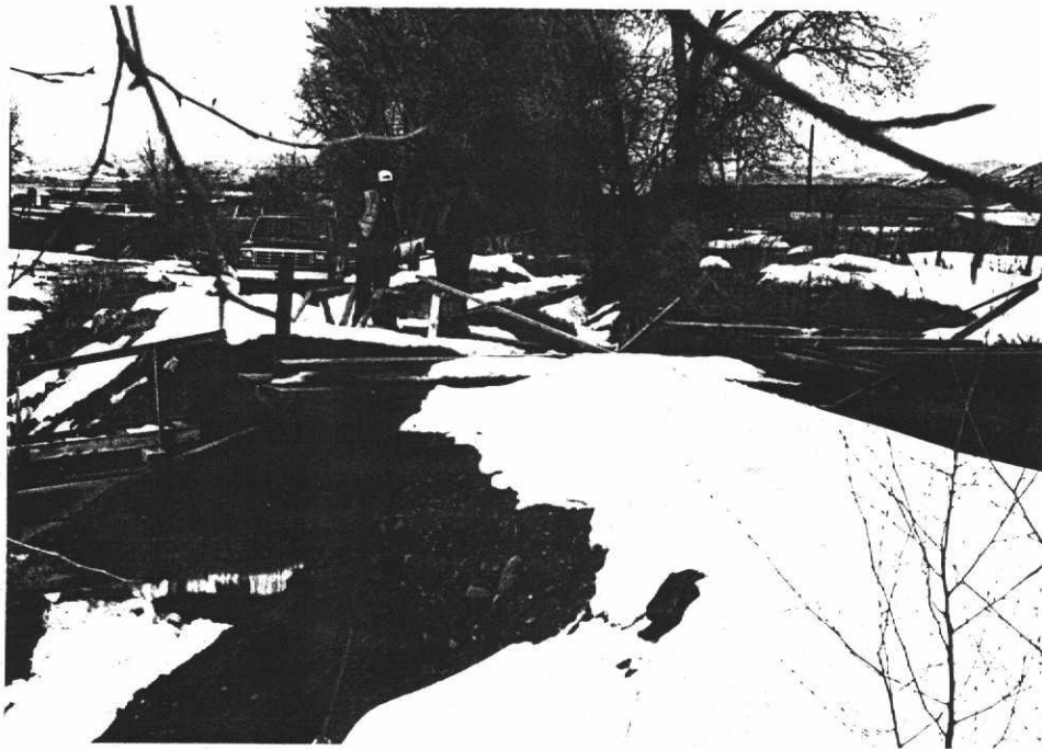
AM lateral irrigation canal spillway severely eroded.
