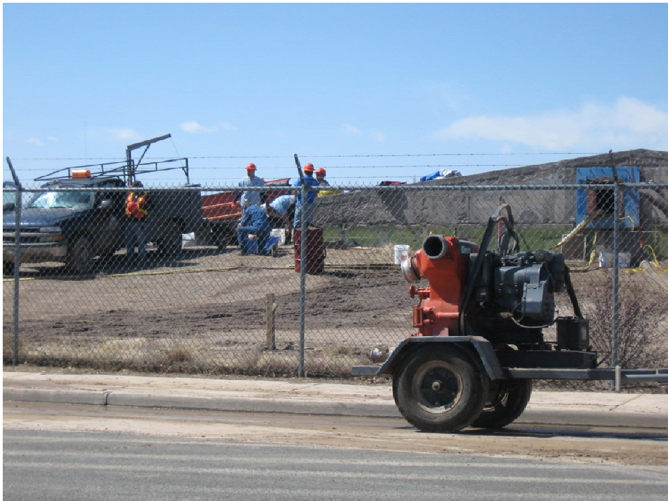
Photo 16: CoWARN crews drained sediment from the Weber Reservoir prior to disinfecting the reservoir with chlorine.
