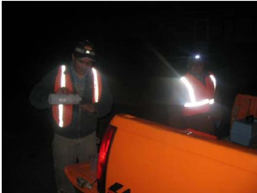
Photo 22: CoWARN crews worked through the night to disinfect and flush all the drinking water pipes.
