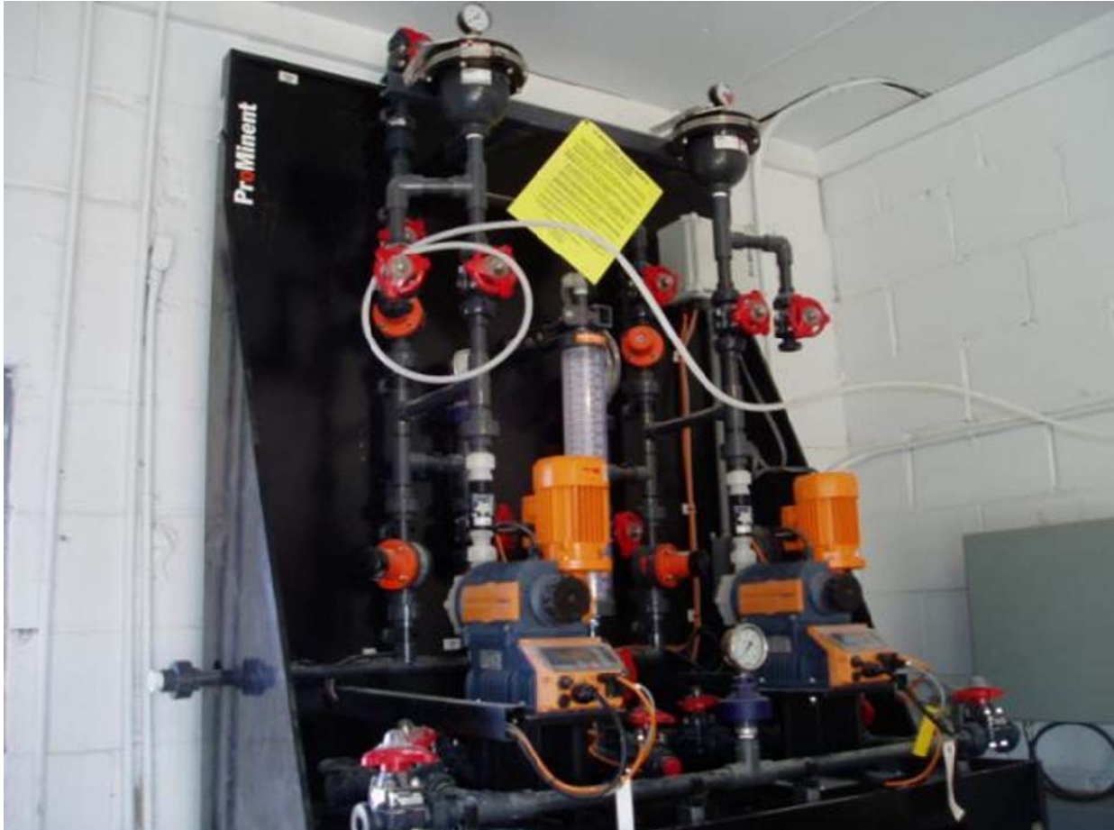
Photo 19: This chlorination treatment unit provided continuous disinfection of Alamosa's drinking water.
