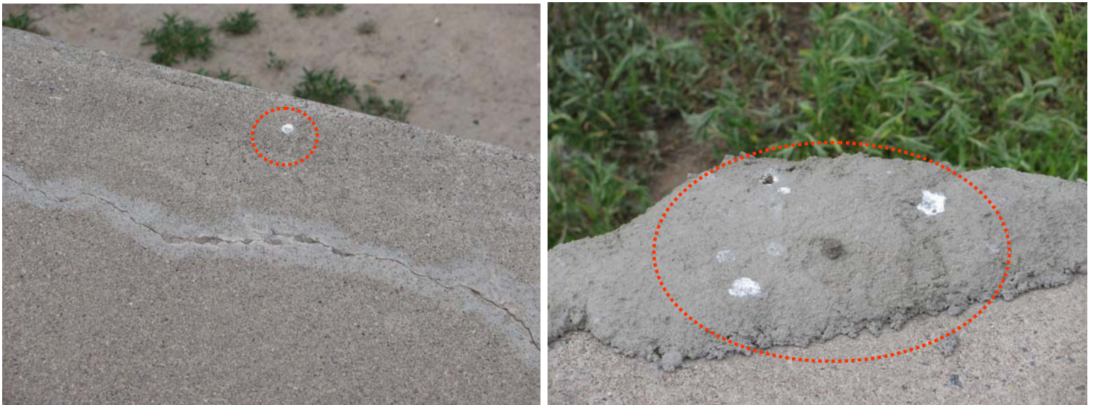
Photo 32: Bird droppings on the Weber Reservoir, including a repaired corner of the reservoir where there previously had been a hole (photos taken in July 2009).
