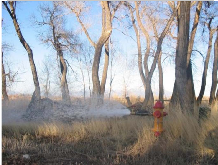
Photo 23: Chlorinated water was flushed throughout the distribution system by opening fire hydrant valves one block at a time.
