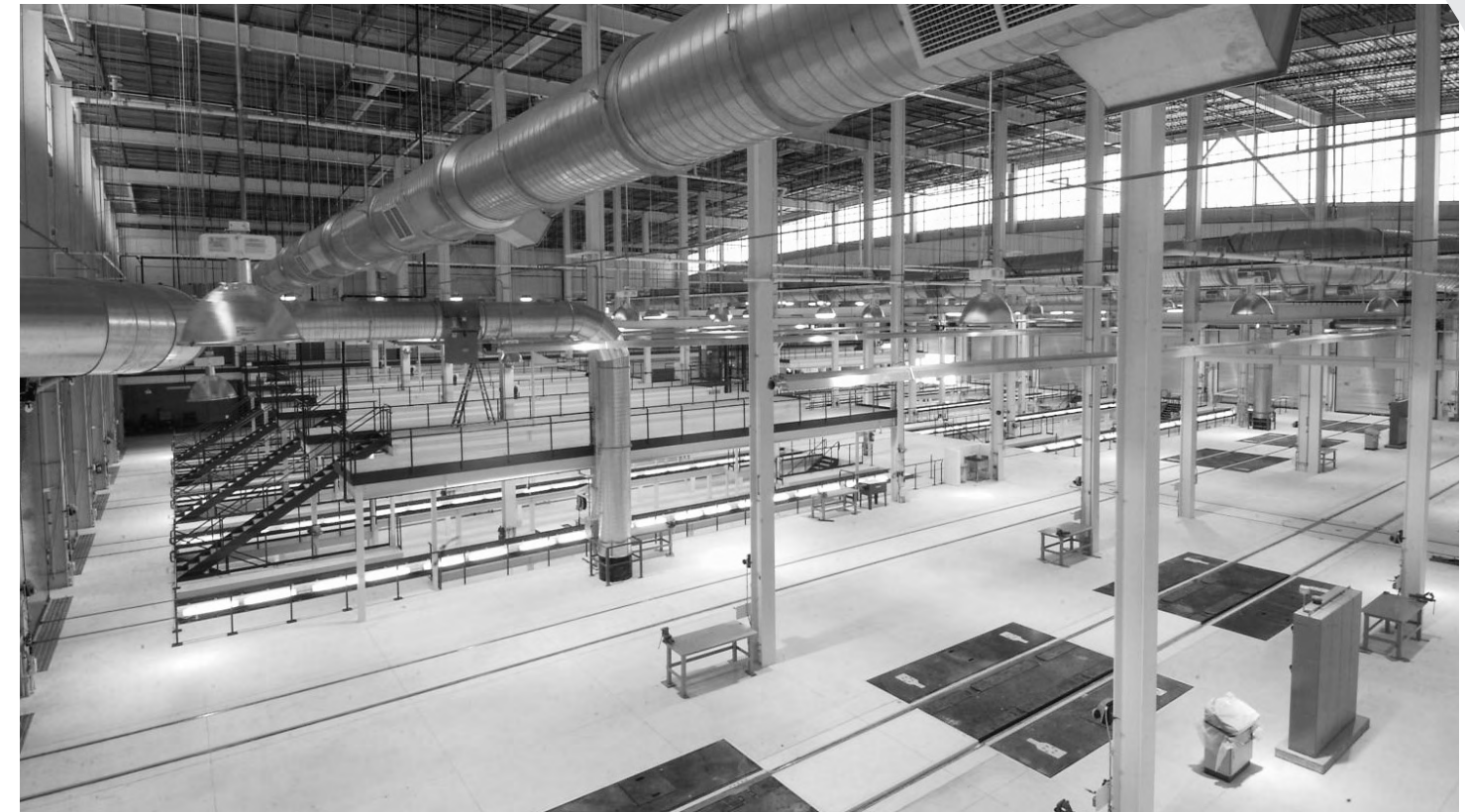
The facility can accommodate 100 vehicles — the number of vehicles that will eventually be a part of RTD's fleet.
