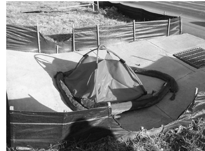
A storm water tent keeps debris from entering the drainage system.
