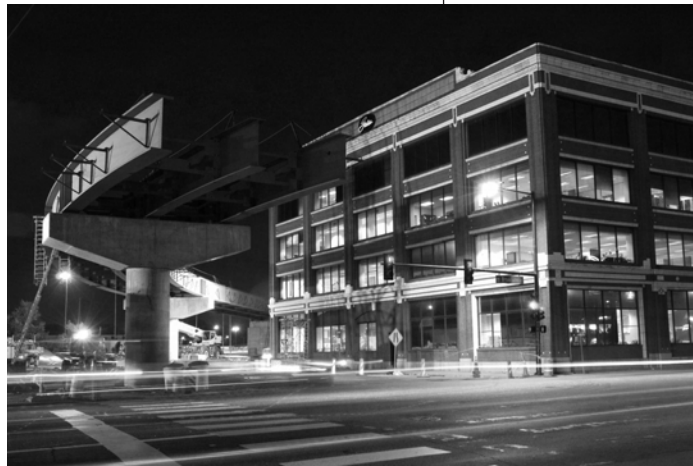
A light rail bridge was constructed over Broadway to connect the Southeast Light Rail with RTD's existing light rail lines.
