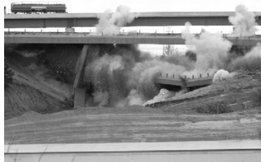
Two bridges were imploded in the I-25/I-225 interchange, making way for new highway and the addition of light rail.
