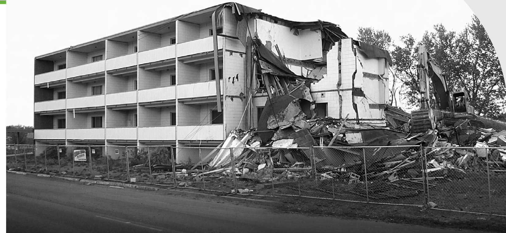
The Woodwinds Apartments were acquired by the right-of-way program, relocating 100+ people. SECC demolished the building to make way for the University of Denver Station and parking garage.
