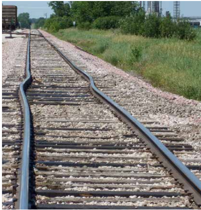
Figure 8.4. High temperatures can lead to rail deformations such as the “sun kinks” seen here on rail lines in Iowa (Photo: Iowa Department of Transportation).
