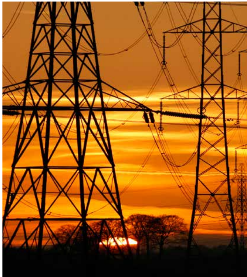
Figure 7.5. As temperatures rise, capacity in transmission lines decreases (Photo: iStock, moonmeister).
