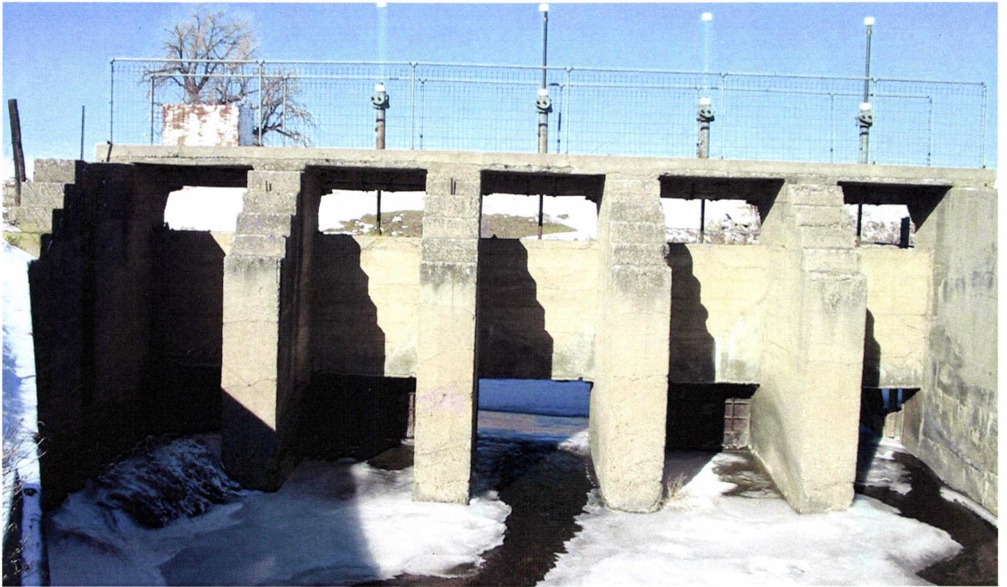
Photo 5 - Big Windsor Diversion - Inlet Gates
