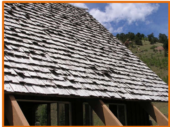
A highly flammable wood shingle roof. Photo: CSFS
