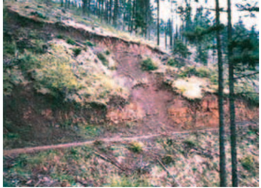
Figure 5-26. Cut-slope erosion example 1.
