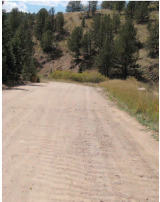
Figure 5-21. Example of poorly maintained road with excessive washboarding. Photo: R.M. Edwards
