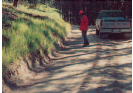
Figure 5-23. The ability of the ditch to handle high-intensity storm runoff from roads; in this case, a roadside ditch is too shallow.
