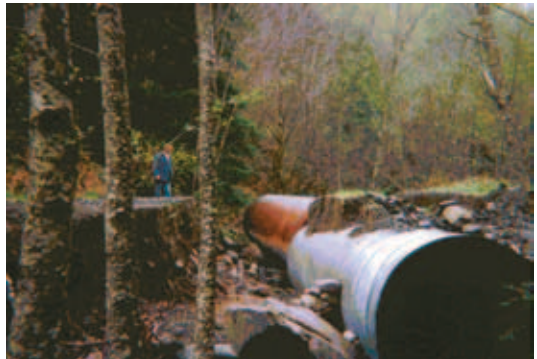
Figure 5-4. Undesired inspection method: inspection of culvert after “blow-out.”
