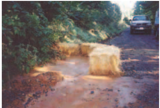
Figure 5-18. Example of road segment without proper water diversion and dissipation methods.
