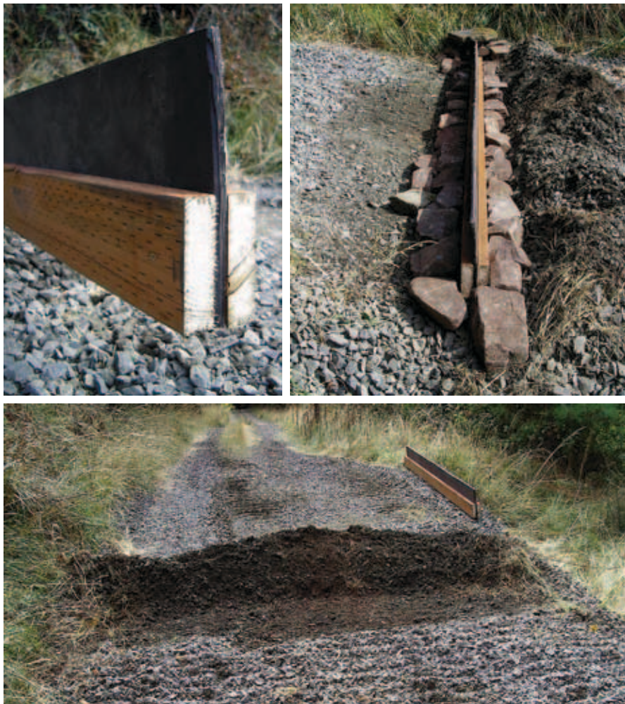
Figures 3-20 through 3-22. Construction details of a laminated 2-inch x 6-inch rubber waterbar.
