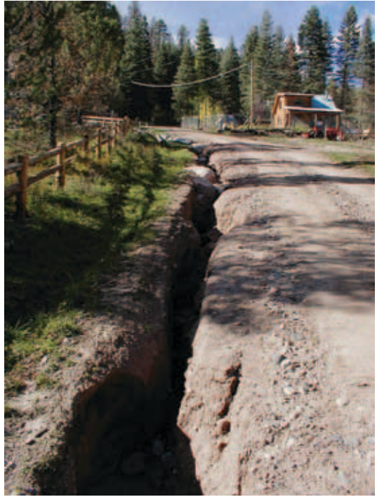
Figure 5-38. Excessive ditchline erosion.
