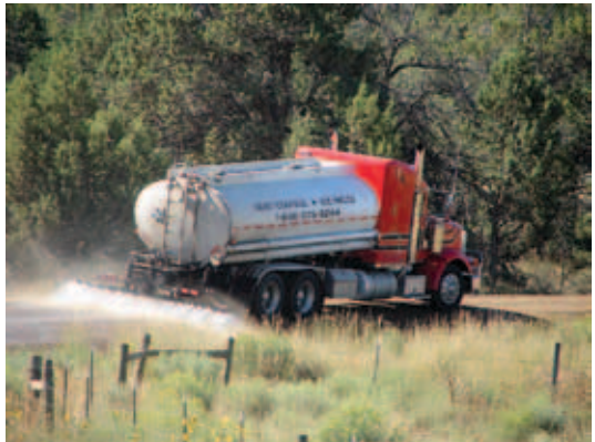
Figure 5-54. Rear view of a dust-suppressant spray truck, illustrating the spray nozzle application apparatus. Photo: Desert Mountain Corporation
