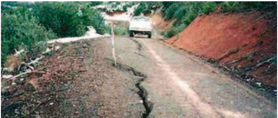
Figure 6-30. Arc-shaped crack on road.
