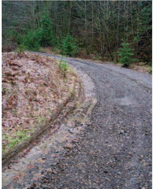
Figure 6-10. Example of road with poor drainage and resulting deformation.
