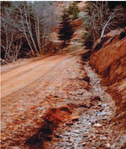
Figure 5-24. Excessive down-cutting of the ditchline likely is the result of too few ditch-relief culverts.
