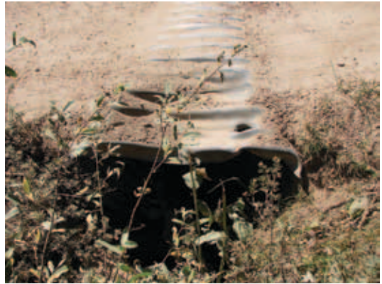
Figure 5-36. Crushed end of steel culvert.
