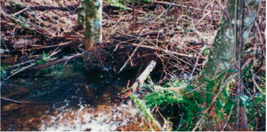
Figure 4-19. Culvert with debris blocking opening.
