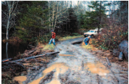
Figure 5-35. Saturated roadbed; the result of a plugged culvert.
