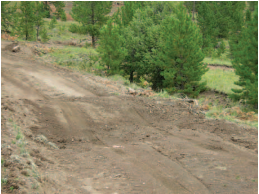
Figure 5-7. Example of a newly constructed waterbar that may require future assessment. Photo: Keb Guralski
