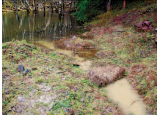
Figure 6-13. Example of delivery of fines from road drainage system.
