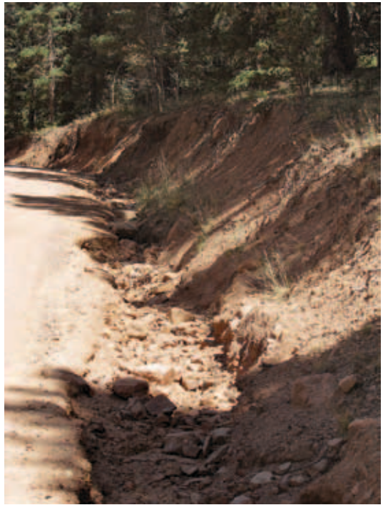
Figure 3-8. Example of a roadside ditch with excessive downcutting. Photo: R.M. Edwards
