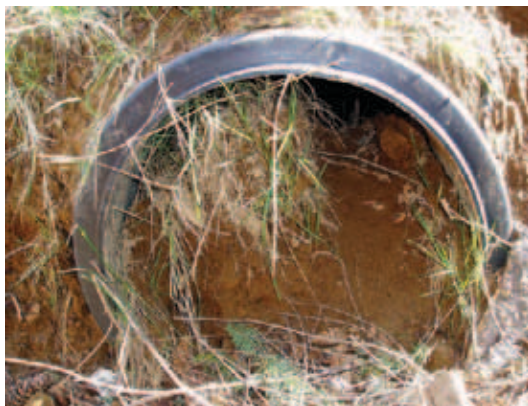
Figure 5-57. Plugged culvert; high priority.
