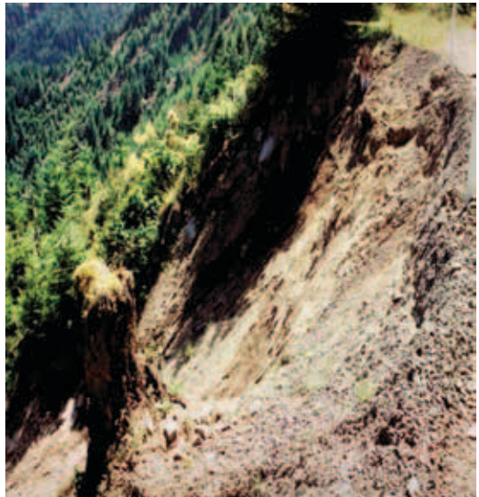
Figure 6-29. Old landslide scar.
