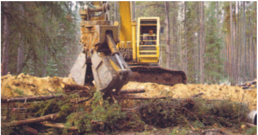
Figure 3-11. A trackhoe compacting/installing slash-filter windrows along the base of a road fill.
