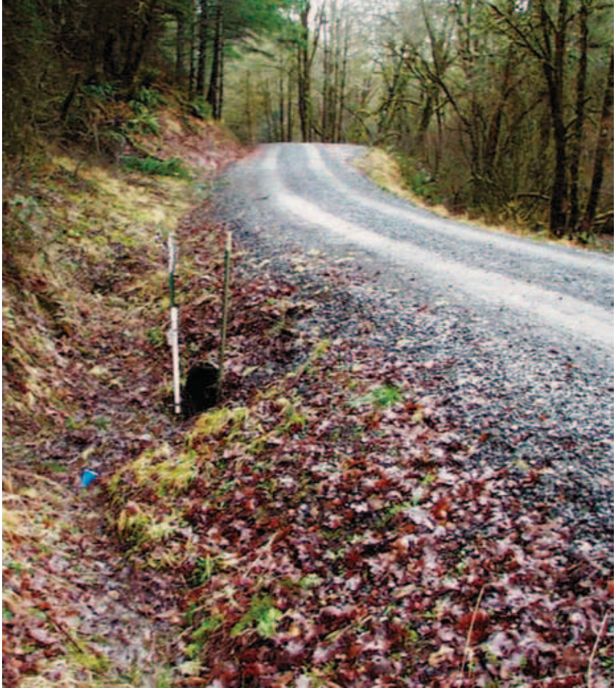
Figure 5-11. T-posts marking culvert location on road for Forest Road Maintenance Needs Form.
