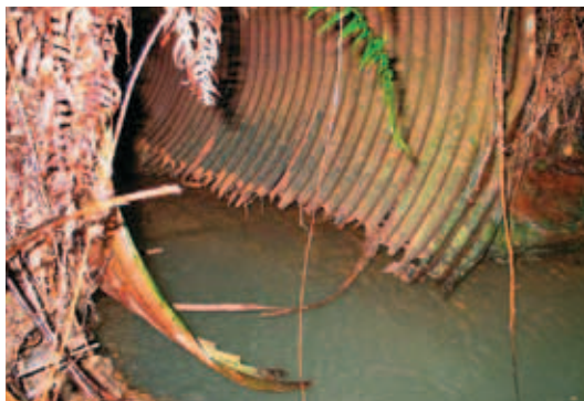
Figure 5-56. Rusted culvert; intermediate priority.
