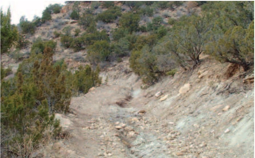
Figure 5-50. Example of a road that may require closure or decommissioning.
