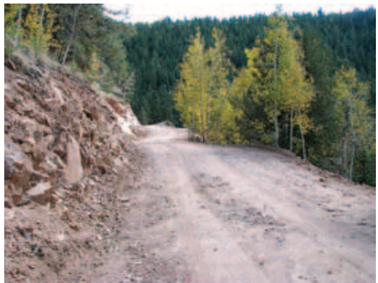
Figure 5-39. Ditchline slumping along cut bank.
