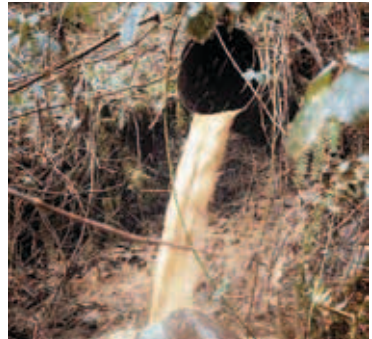
Figure 5-40. Example of a culvert contributing to downslope erosion.
