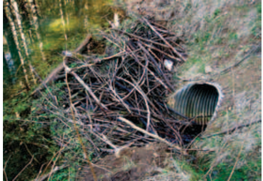
Figure 5-34. A partially plugged culvert.
