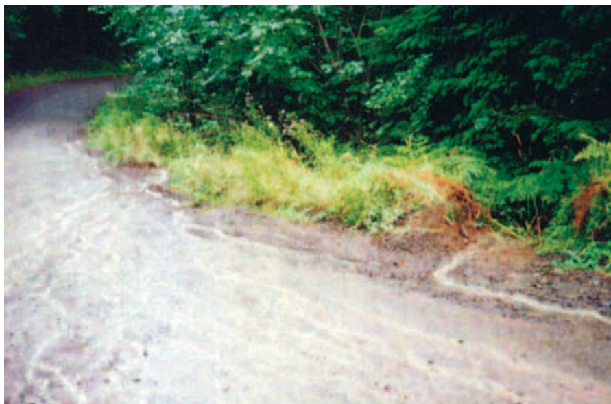
Figure 6-23. Example of a road that has become a drainage channel.
