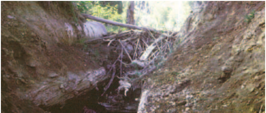
Figure 4-21. Washout caused by culvert failure.
