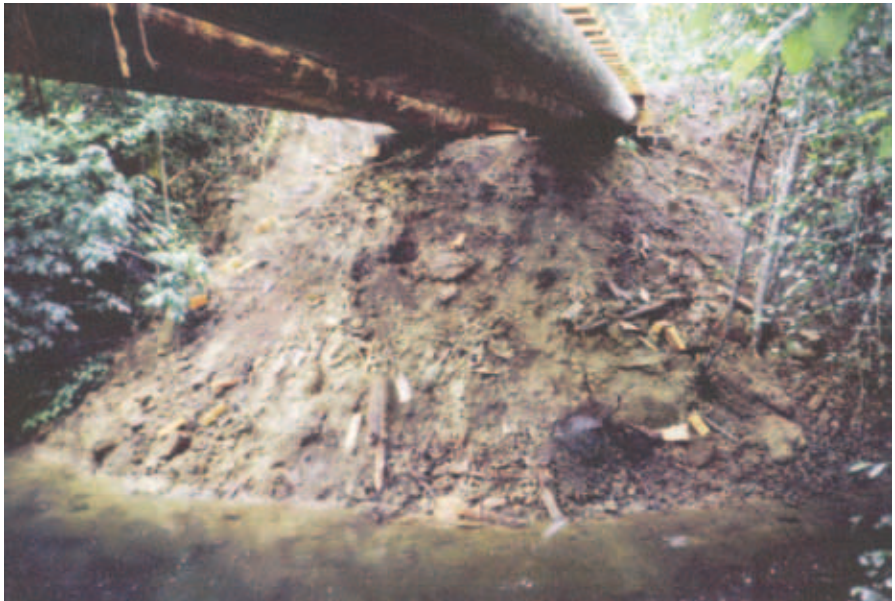
Figure 5-1. Exposed bridge-fill next to stream.
