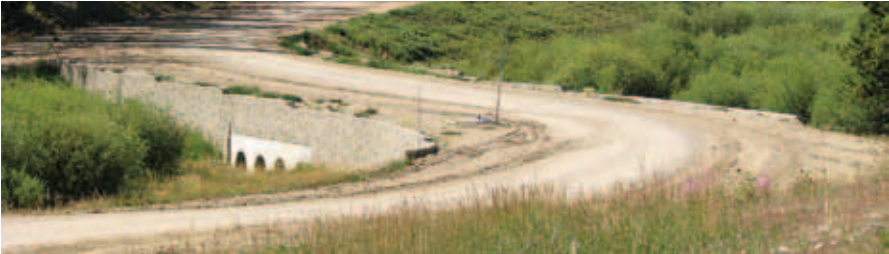
Figure 4-15. Example of a multiple culvert crossing with decorative retaining walls. Photo: R.M. Edwards
