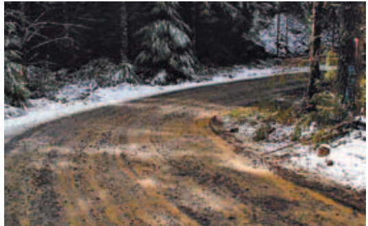
Figure 6-14. Example of a poorly surfaced road.
