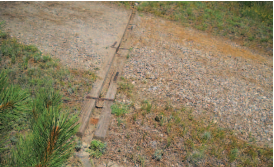
Figure 5-14. Example of priority repair involving a wood culvert. Photo: Dan Wand
