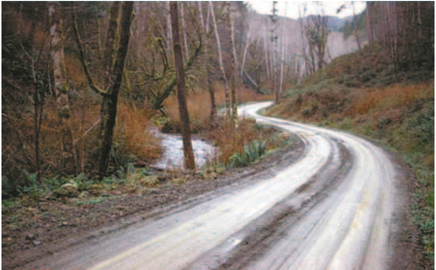
Figure 6-12. Example of a road adjacent to a stream with inadequate surfacing.
