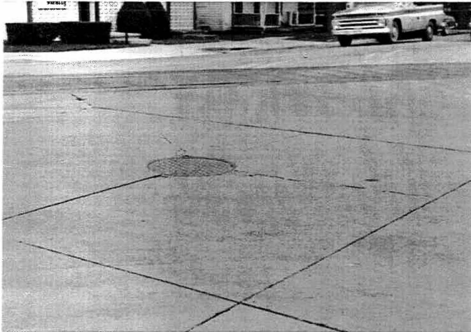
Photo 4: Formation of diagonal cracks due to presence of manhole and/or irregular joint spacing.
