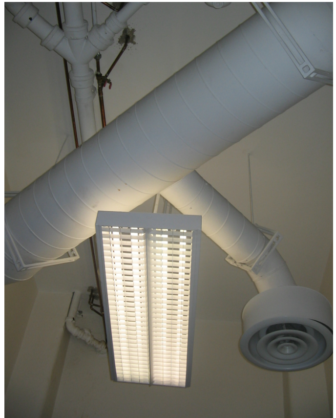
060 Exposed MEP over-head
