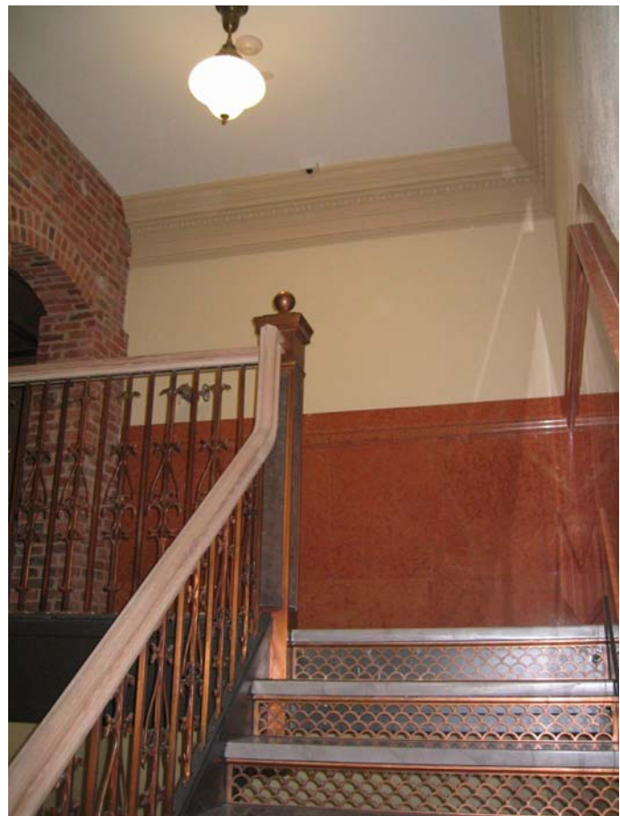
New landing at Attic looking south, prior to finish being applied to handrail
