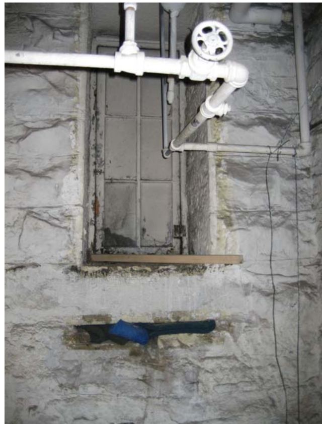
Failed mortar joint at Sub-Basement
