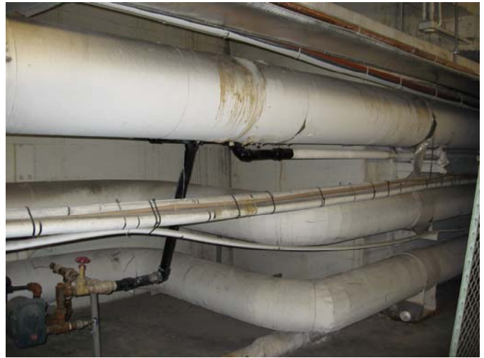
East Tunnel steam lines
