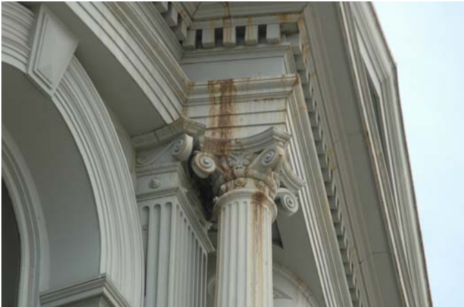
Corrosion at column capitol
