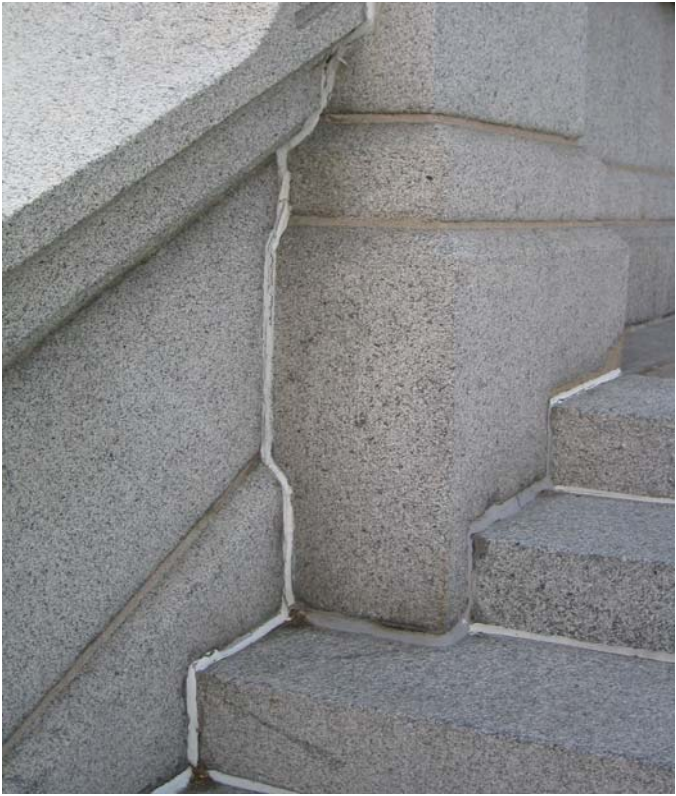
Incorrect caulk joints at steps
