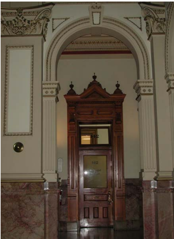
Public corridor door showing typical trim type T5 with original door glazing and non-original clear transom glazing
