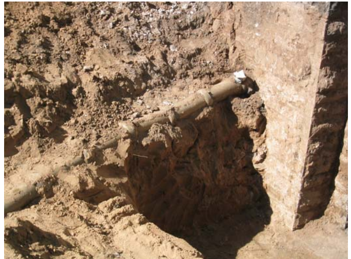
Excavation of drain leader at north east area well location. This pipe section
