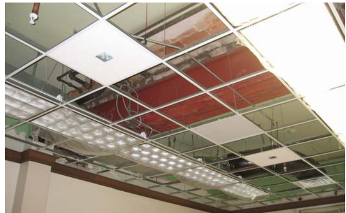
0111 View above ceiling at steel beam added when masonry wall was removed during 1968 remodel
