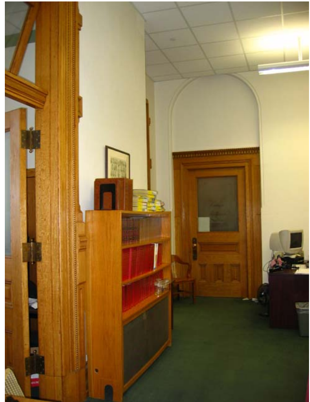
346 In-filled archway with missing wainscot
