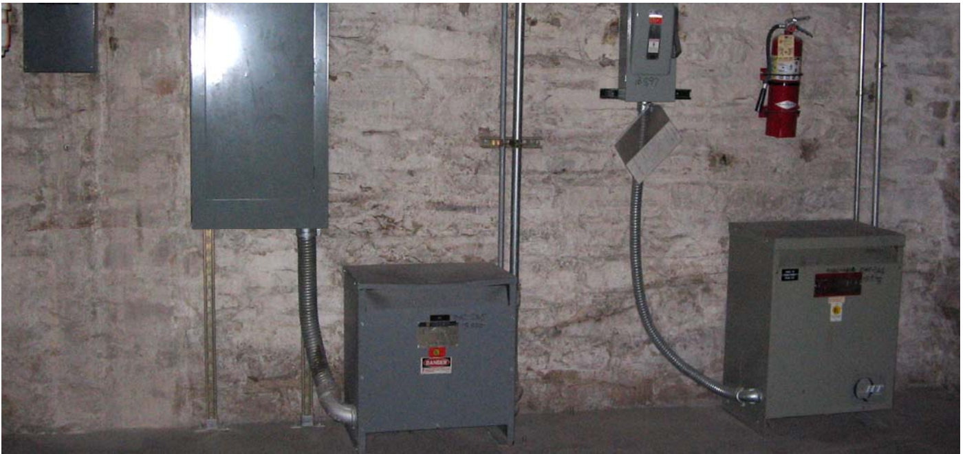
Transformers in Sub-Basement
