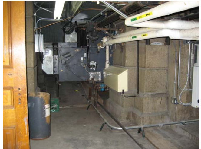
0116 View south at air handling units
