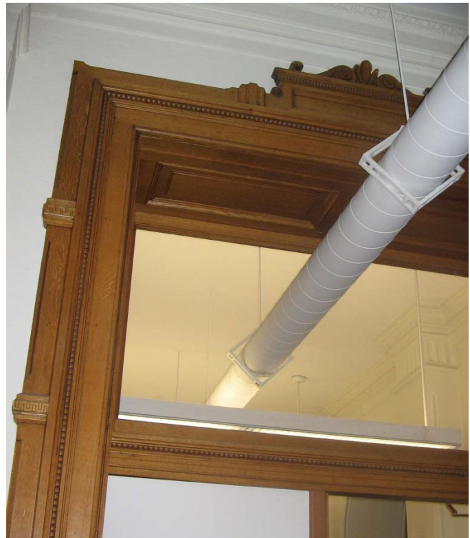
083 Exposed duct and missing transom glass
