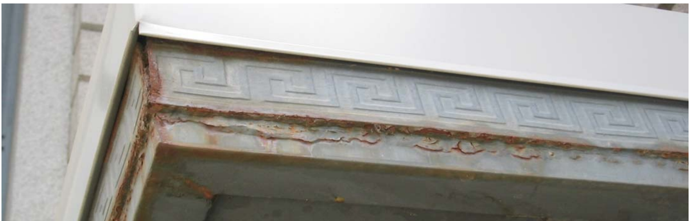
Rust on fascia above Basement entries
