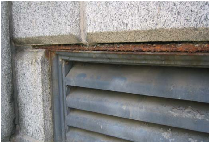
Rusting mechanical vent
