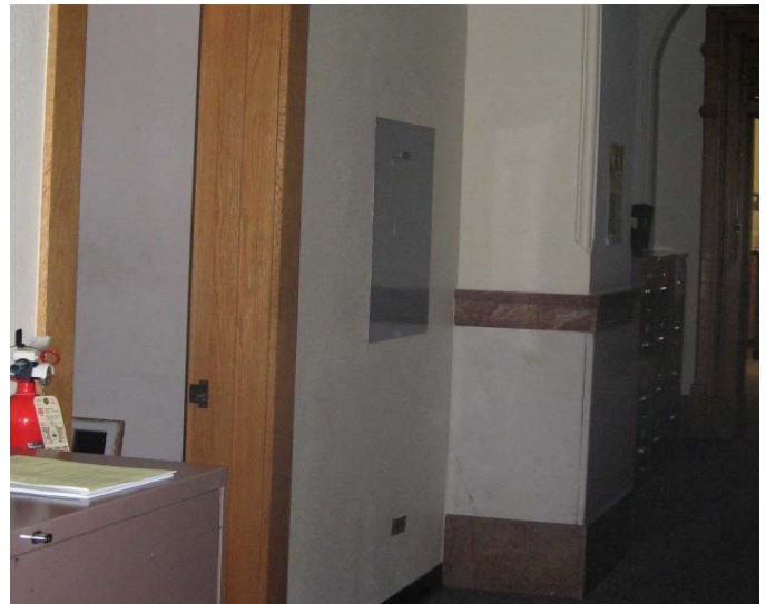
088 Wainscot discontinues after wall intersection
