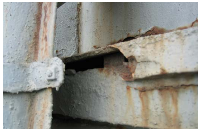
Broken cast iron behind downspout
