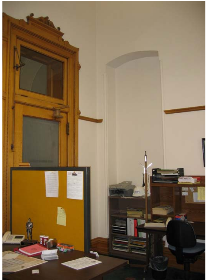
305 Arched in-fill on northwest corner; formerly an access to what was once a laundry area
