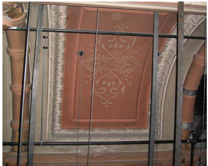
Attic: Senate Chamber Skylight, hand painted panel
