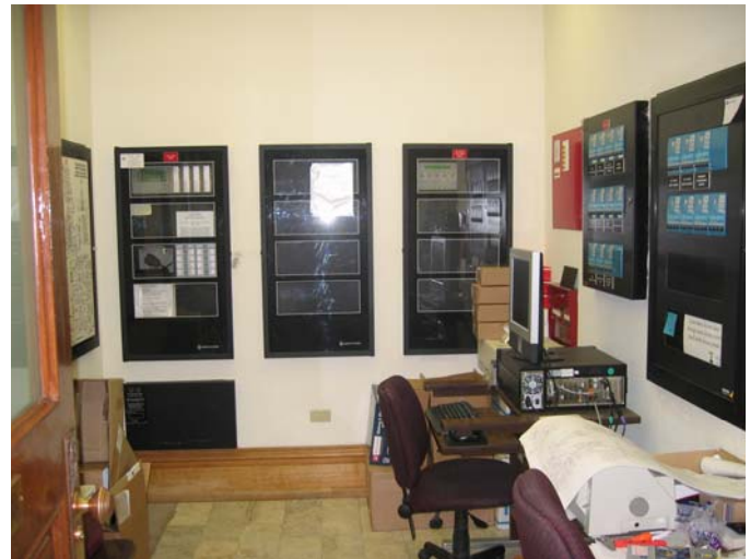
078 fire alarm panels
