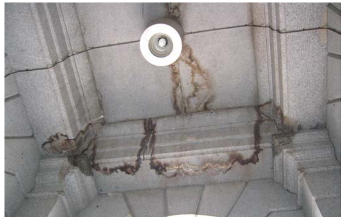
Stains at East Portico from water collecting on the porch above
