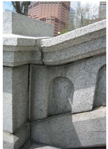
West Steps open joint resulting from settling
