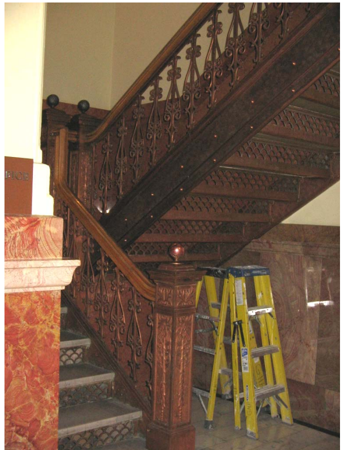
Existing stair and landing at Second Floor; bottom landing will be partially
