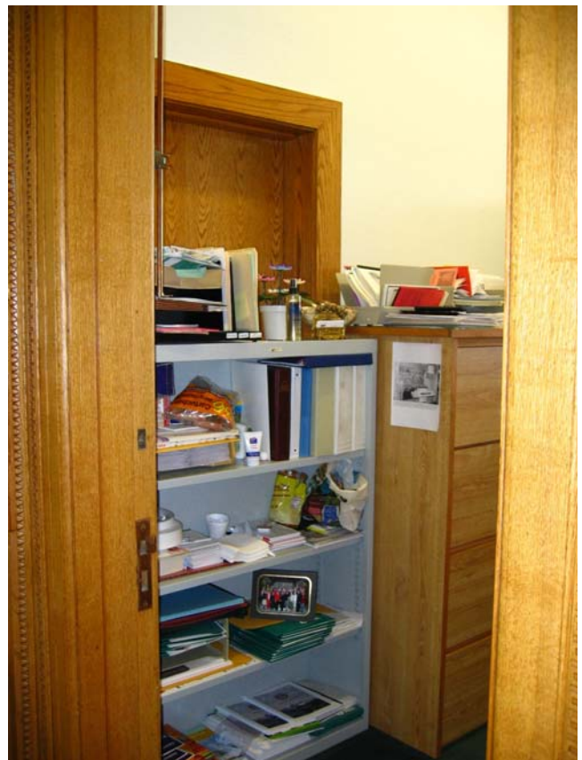
347 View of inoperable connecting door to Room 348
