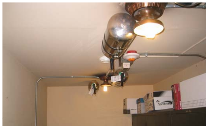
140B FM200 Fire extinguishing system inside modified vault 140B
