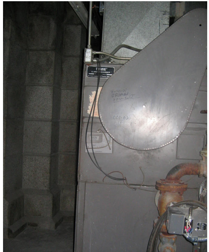
052 AHU in former breezeway
