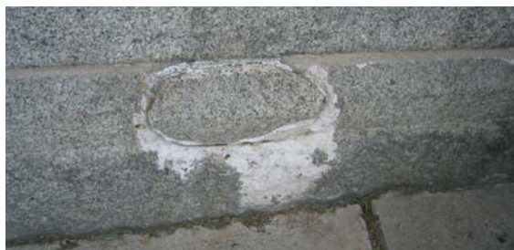
A poorly executed patch
