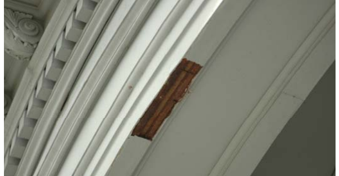
Cast Iron façade damage from winter 2005
