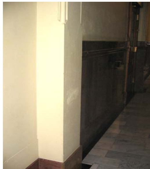
328 Missing wainscot at east wall archway
