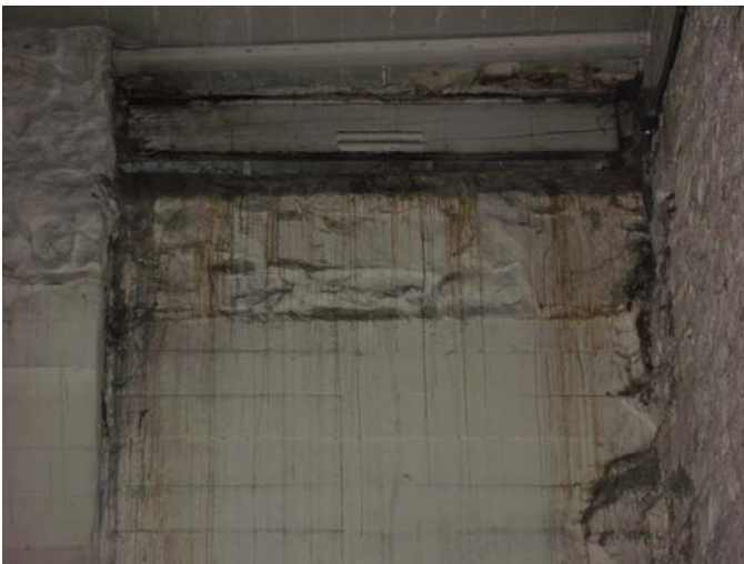
East Tunnel water damage and decaying ceiling structure
