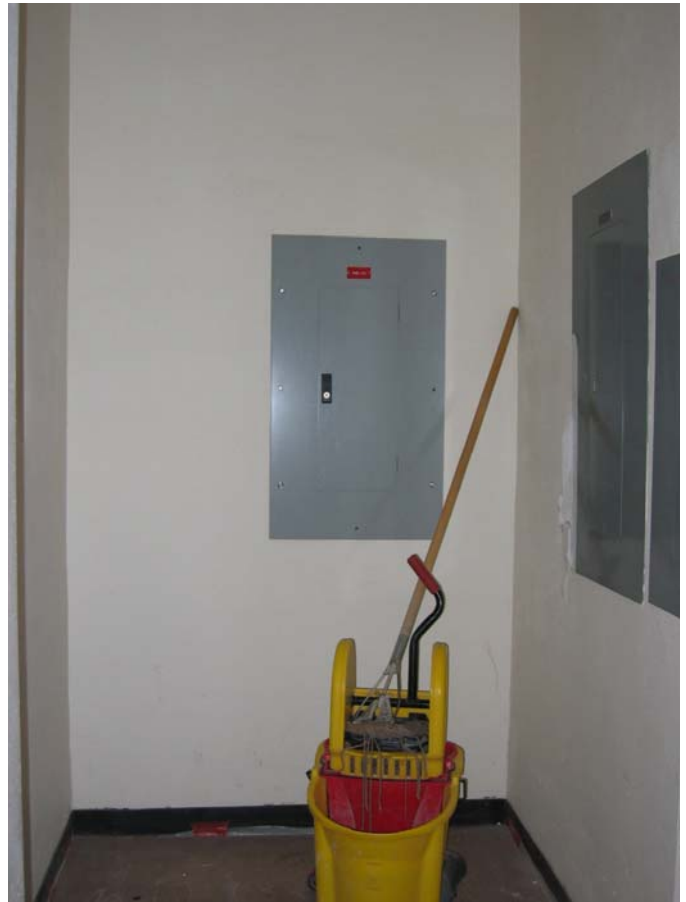
110A South wall view of electrical panels
