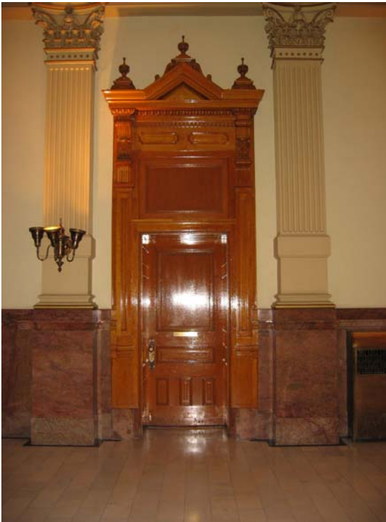
Public corridor door showing typical trim type T5 with non-original wood panel at door and transom
