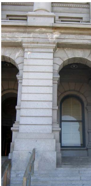
Lime stains at porch
