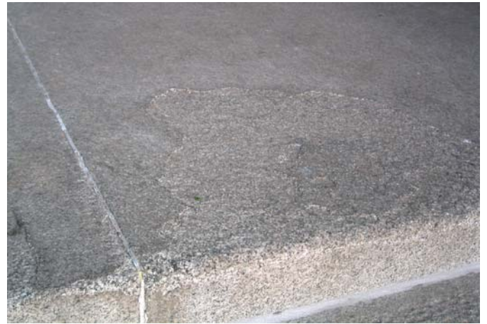
Granite spalling at East entry
