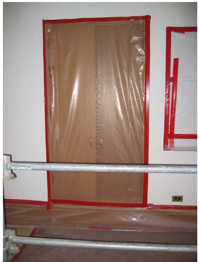
103 Cabinet on west wall protected during phase 3 of the 2006 Life Safety Project
