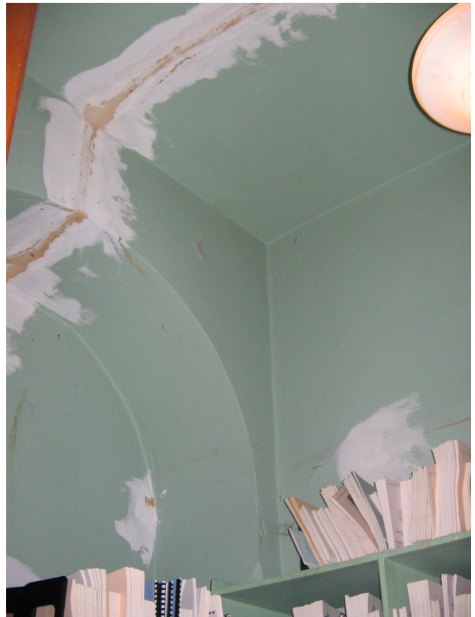
018 In- filled arch opening and poorly patched crack in the plaster
