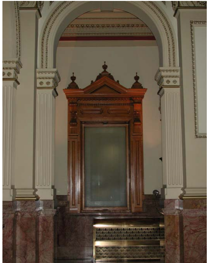
Existing window and radiator enclosure, prior to removal at First Floor Northeast Stair
