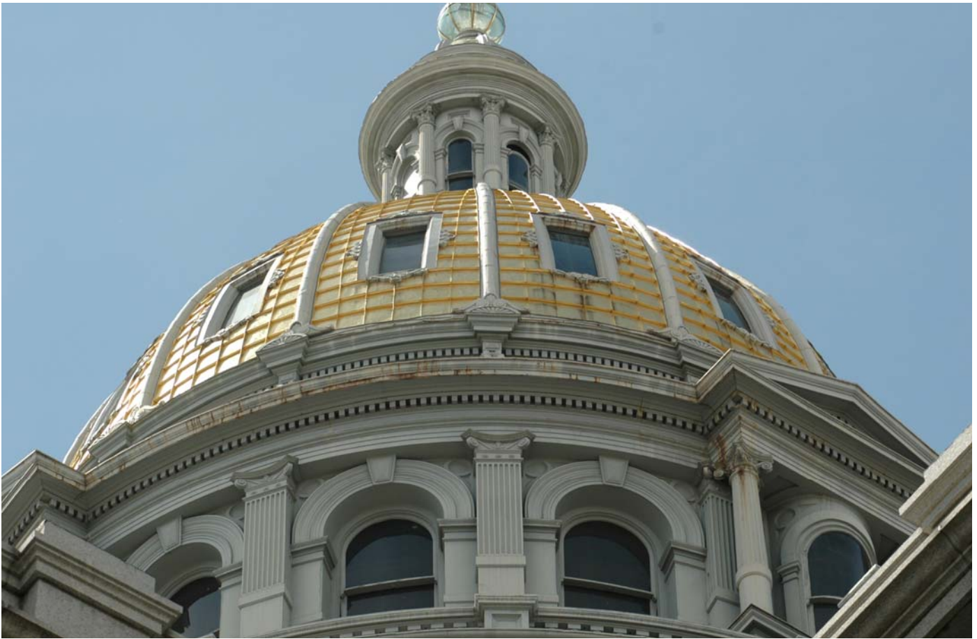
Staining from corrosion on columns and ledges at Dome windows
