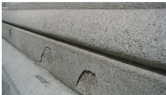
Example of spalling
