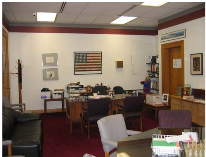
266 North wall with access panel to mechanical chase in the east corner
