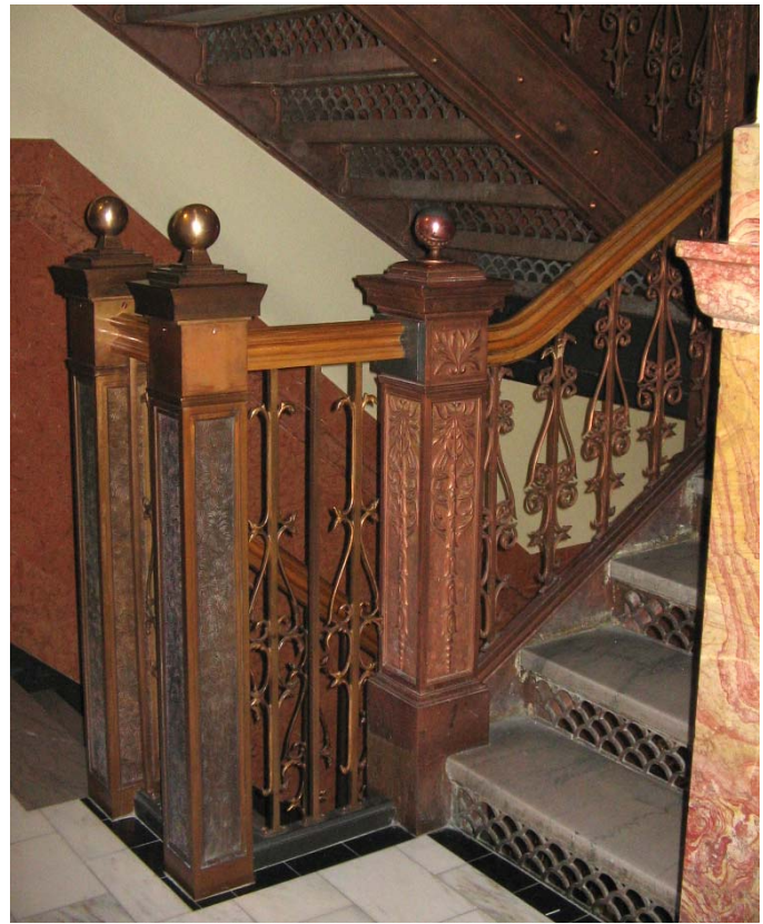
Transition of Northwest Stair from existing to new at the Second Floor
