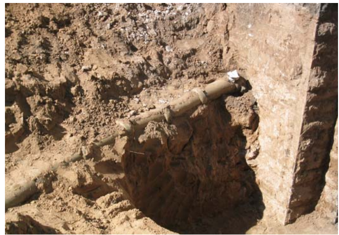
Excavation of a drain leader at north east area well. This pipe was replaced, but the condition is typical of drain leaders around the building
