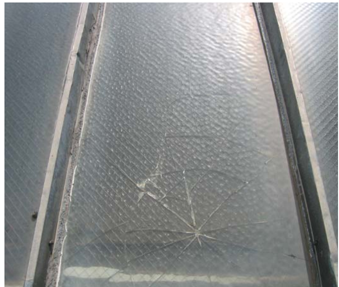
Cracked skylight glazing
