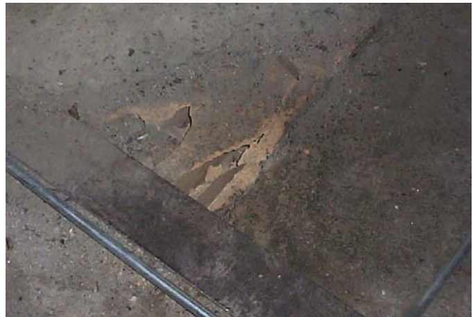
Attic: Chipped concrete floor exposing broken terracotta structure
