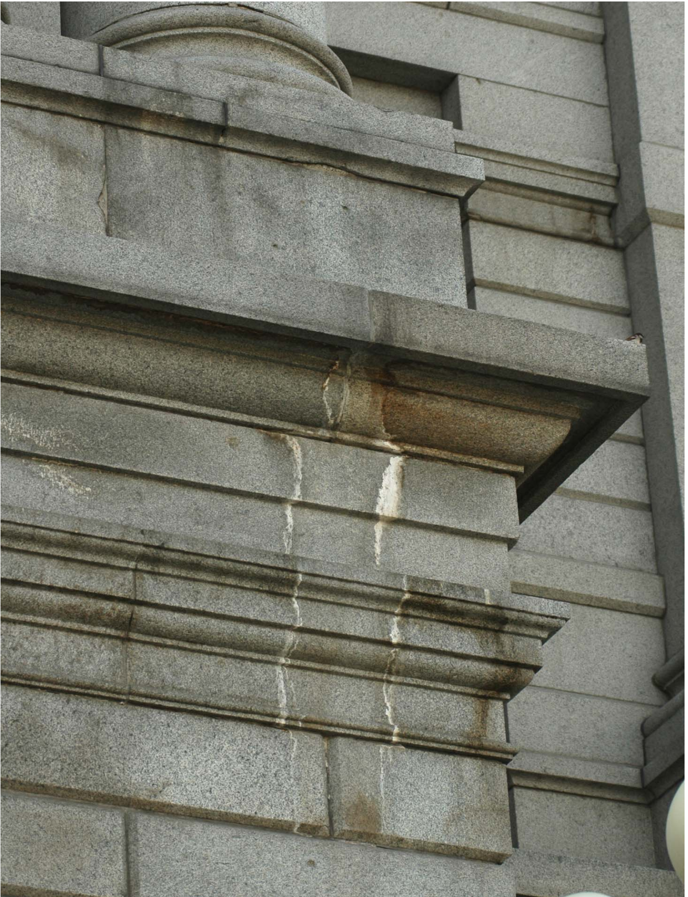
Lime stains on granite facade
