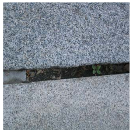
West Steps open joints
