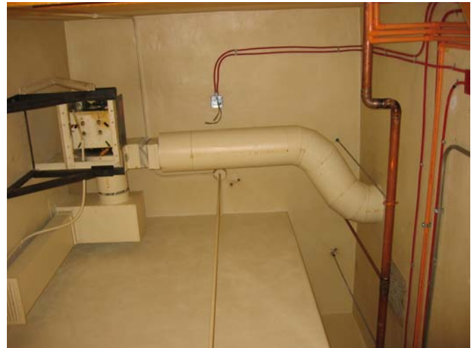
116 Ceiling with exposed MEP systems
