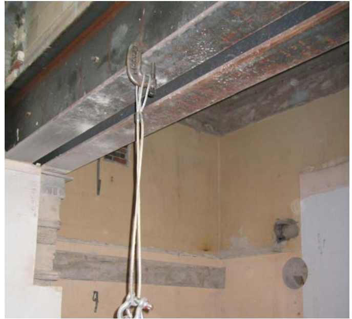
Steel beams where wall was removed with work for new Basement Northwest Stair in background
