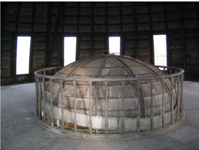
Upper Dome: Steel plate floor and cap of inner dome w/cast iron guardrail
