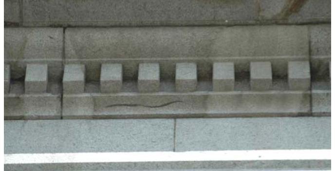
Horizontal crack in carved granite
