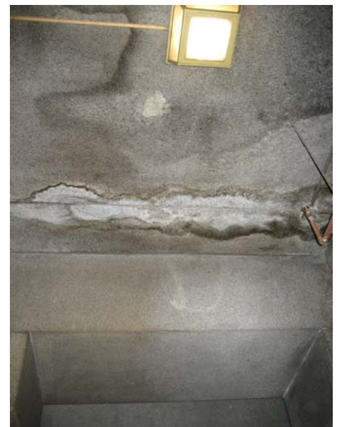
051 Water damage on ceiling
