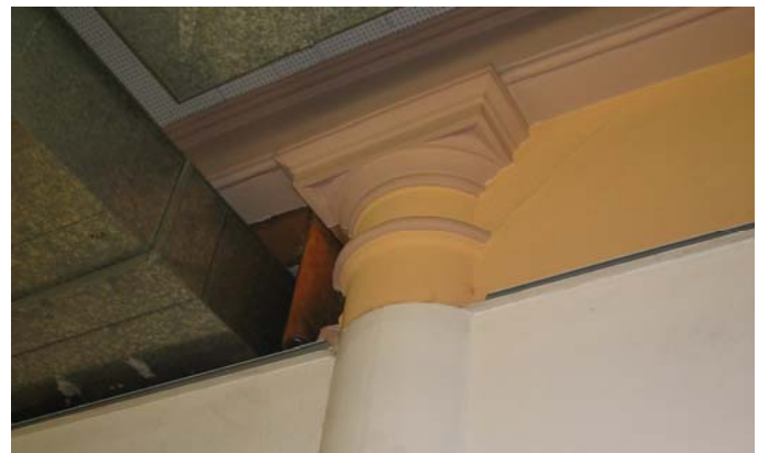
027 Free standing column now engage in non-original wall
