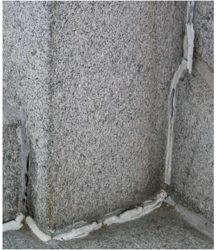
Failing caulk joints
