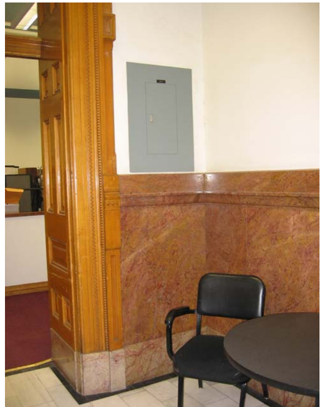
127 Electrical panel in south east corner
