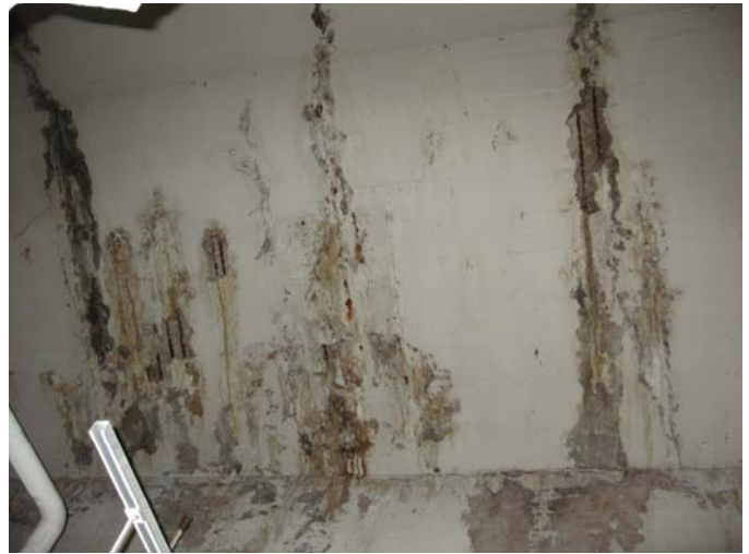
East Tunnel decaying ceiling structure
