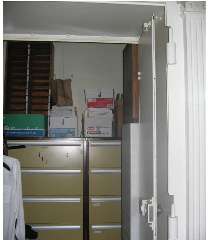
105A Hinge pins for missing vault door
