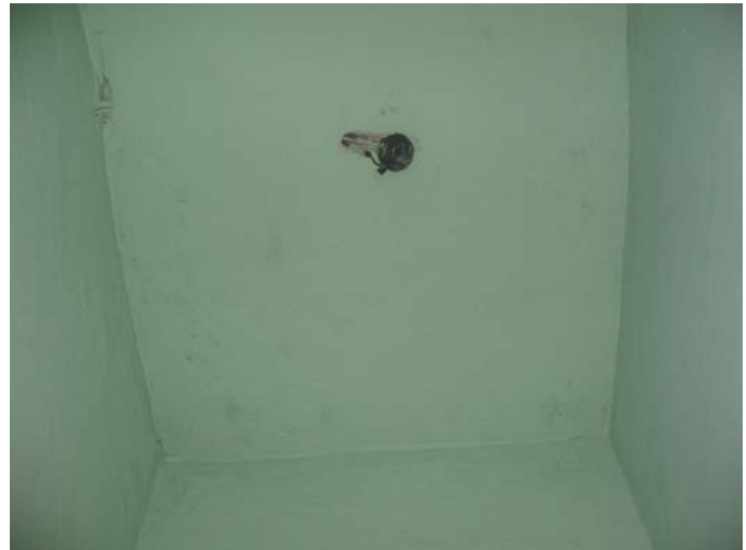
013 Exposed wires and missing light fixture
