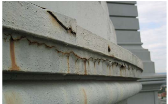
Broken and corroded cast iron
