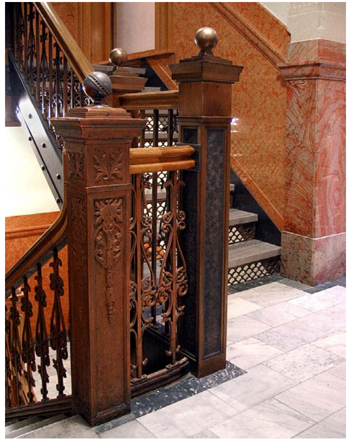
Stair transition at Third Floor landing with original newel post on left and new newel post on right
