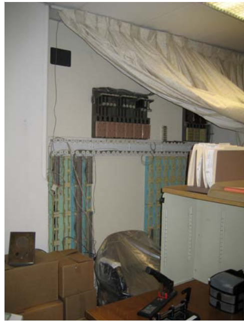
054 Existing telecom board
