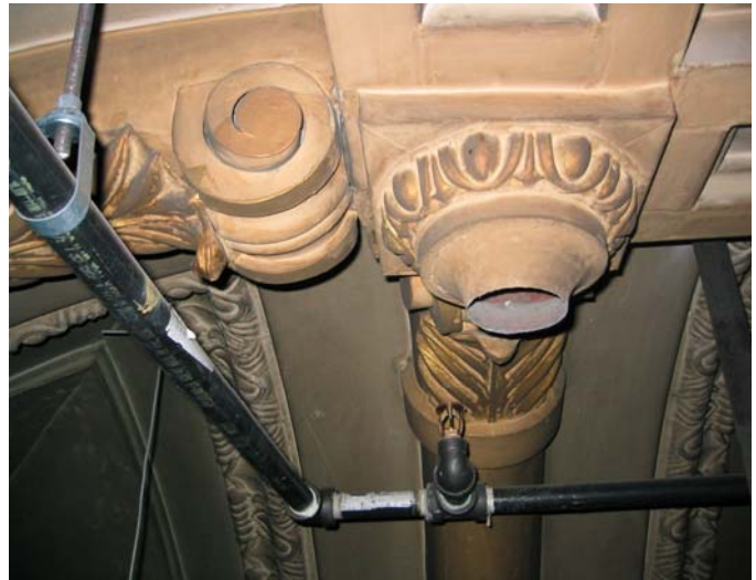
Attic: Senate Chamber skylight missing pendant
