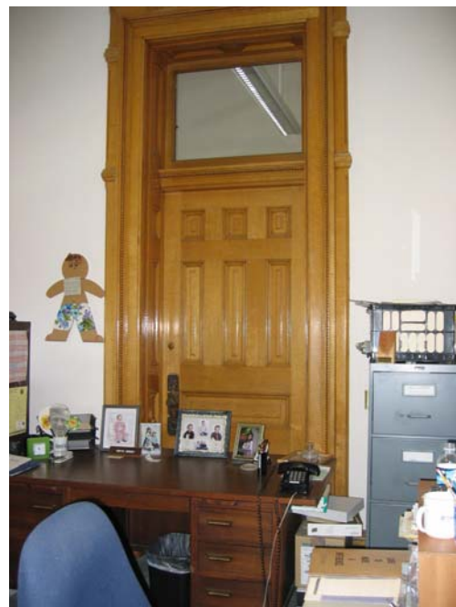
320 Interconnecting door to Room 322; inoperable
