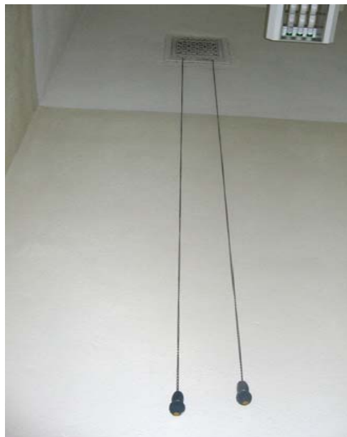
304 Original damper operator in place
