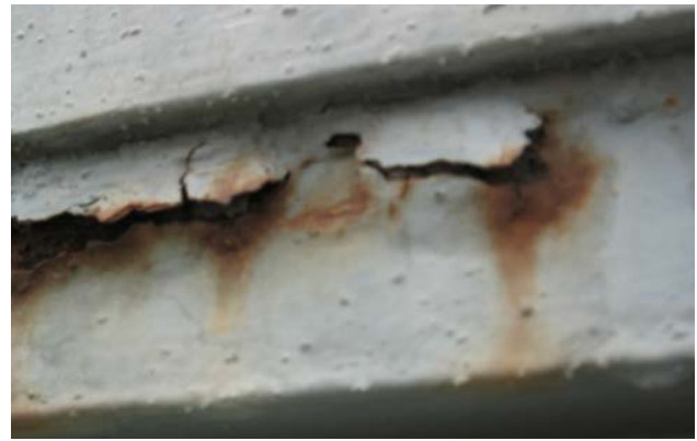
Corrosion above the drum
