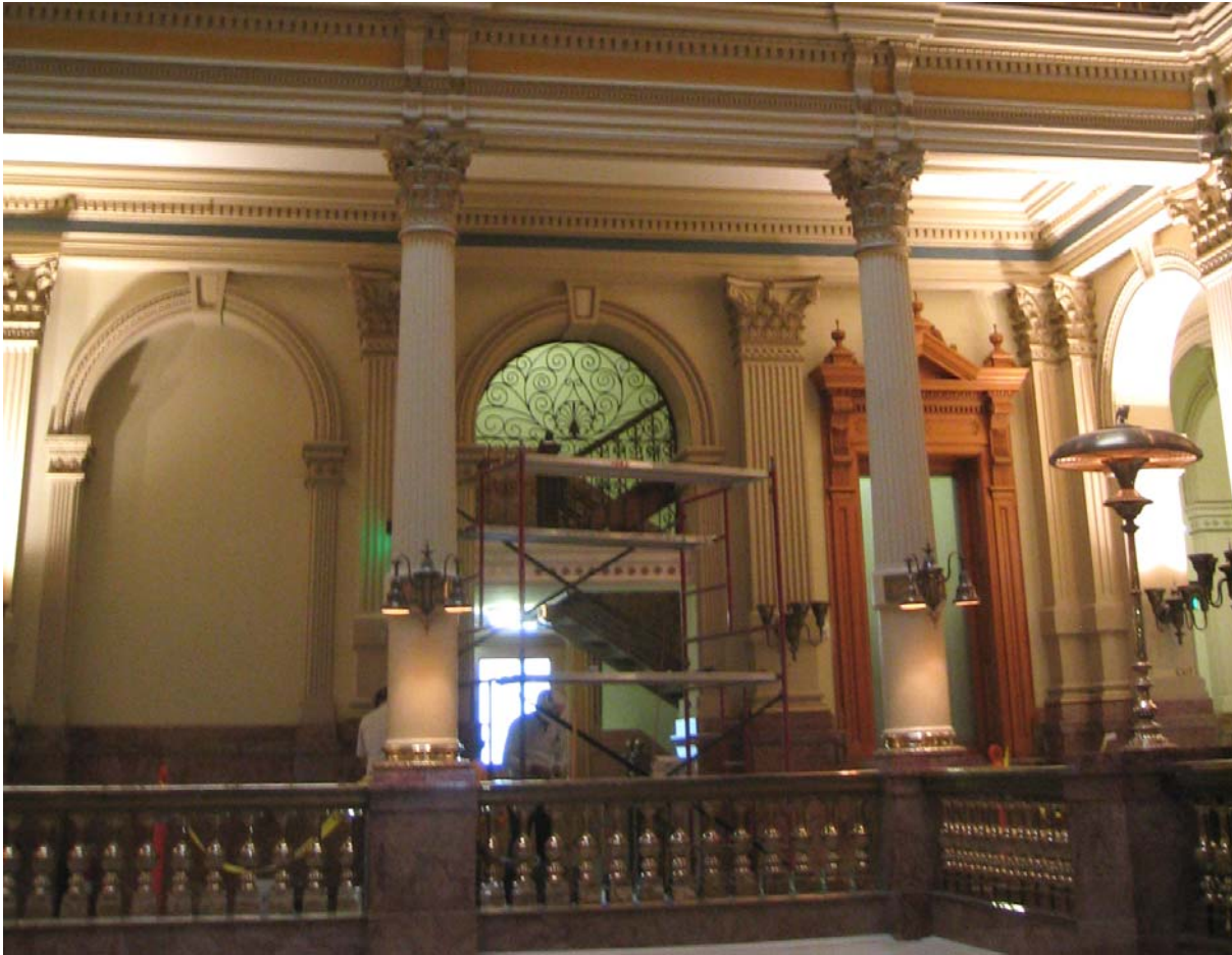
Overall view of the north Arcade at the Second Floor during construction of the North West Stair
