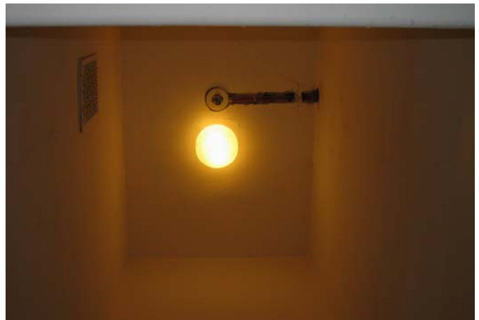
110A Ceiling showing lighting and smoke detection channeling as part of the Life Safety Project
