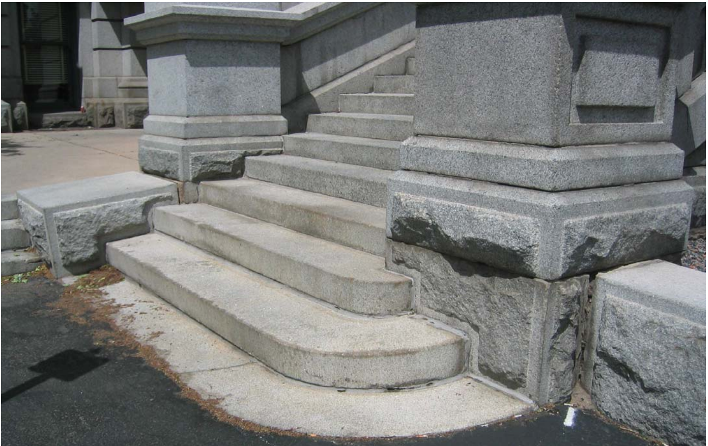
Settling at South Steps and features, caulked joints
