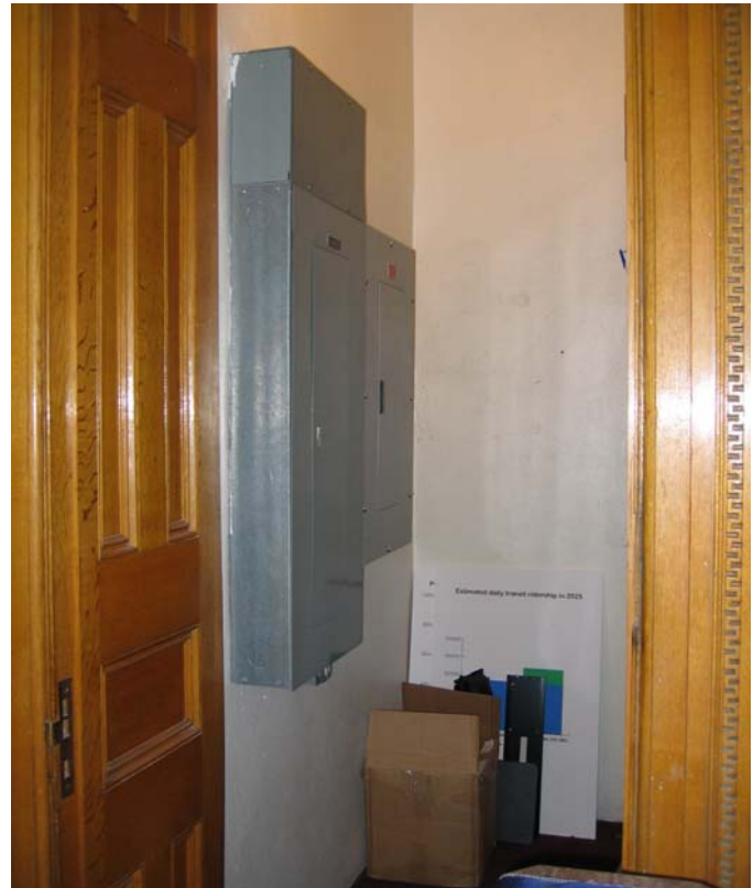
124A West wall with view of electrical panels
