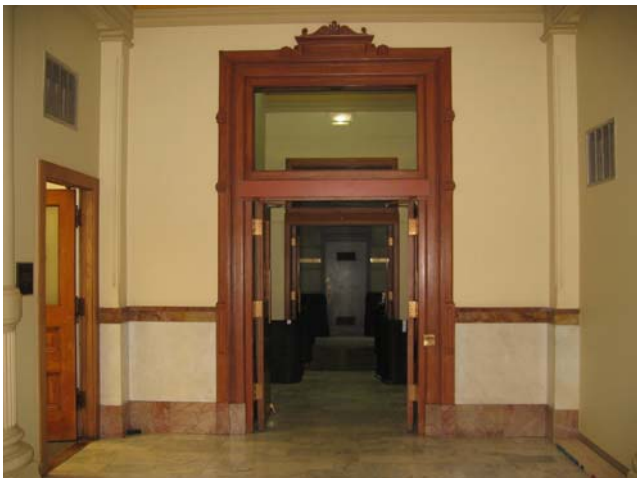
Remaining South Entry Vestibule door
