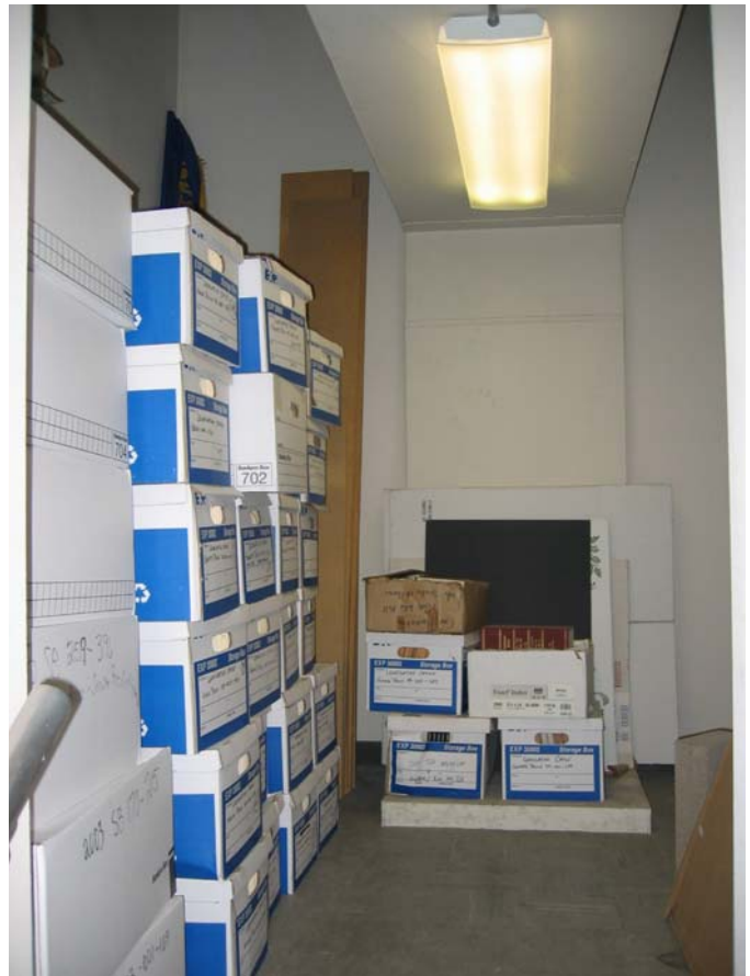
128B Duct along north wall with surface mounted light fixture
