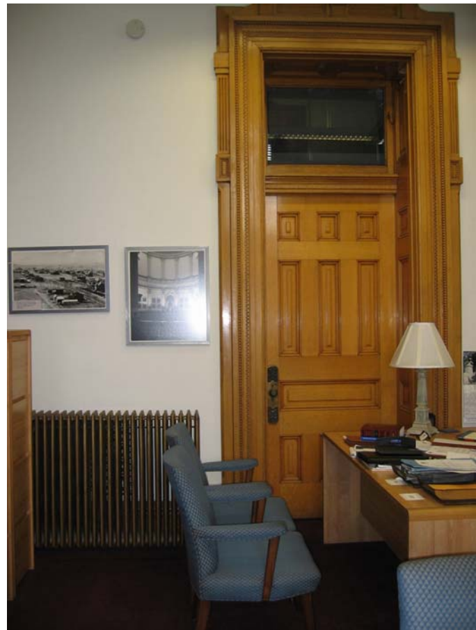
121 Freestanding radiator outside interconnecting door to 120A
