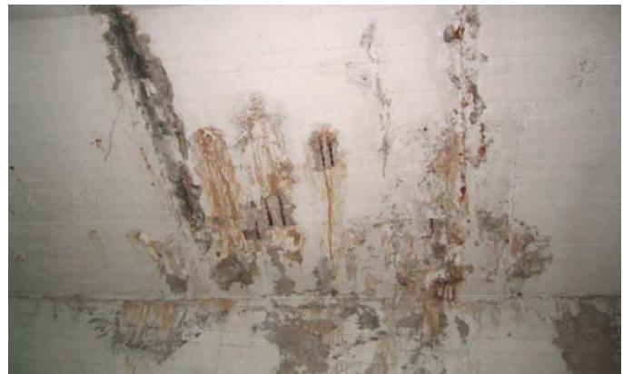
Decaying concrete and reinforcing below the East Steps
