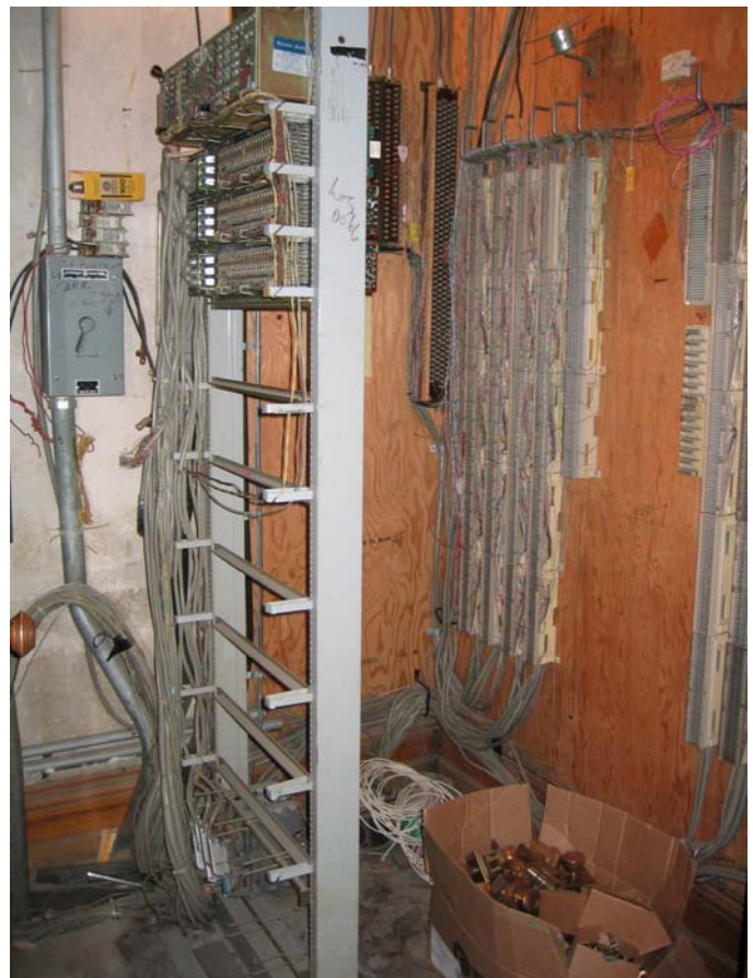
137 Existing electrical panels and telecomm equipment
