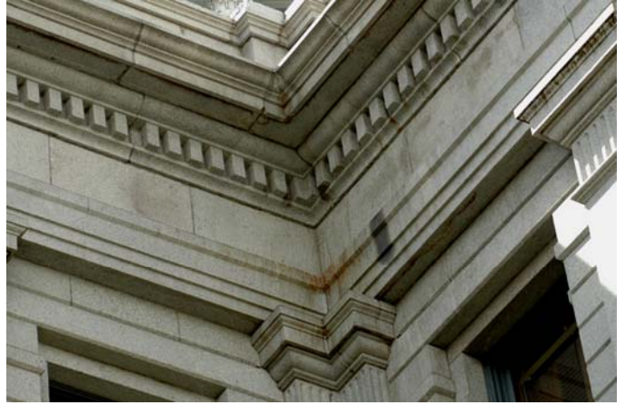
Staining and failed joints
