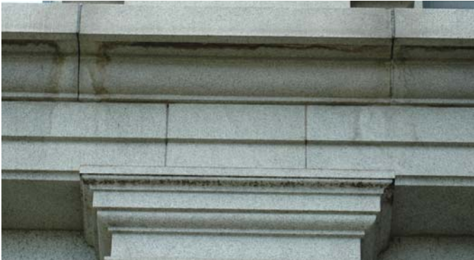
Lime staining at failed joints
