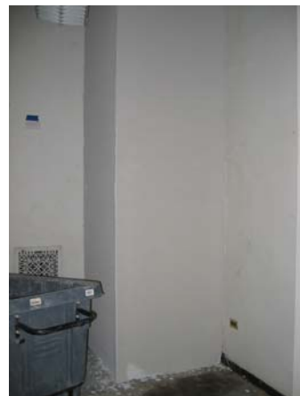
016 Pressurization duct enclosure
