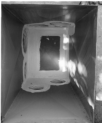
Sealing plenums: Sometimes you need to cut an access hole to seal a plenum properly.
