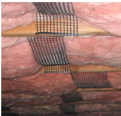
Nylon mesh: This floor insulation is held up next to the bottom of the floor by nylon mesh, stapled in place.
