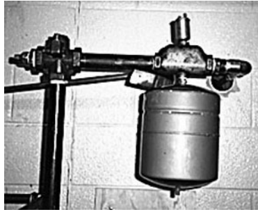
Pressure tank, air separator, and vent
