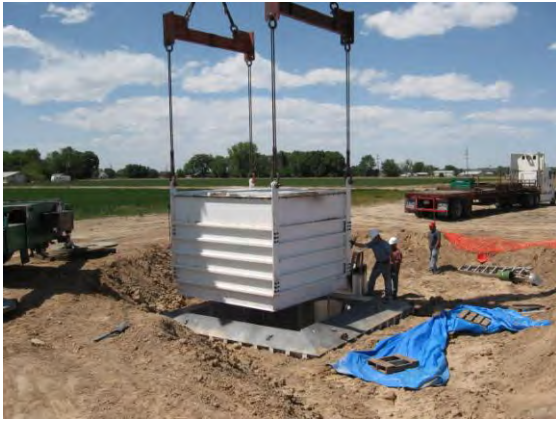
Figure 2. The inner tank plus soil being lowered inside the containment tank. Photo taken by Michael Bartolo.
