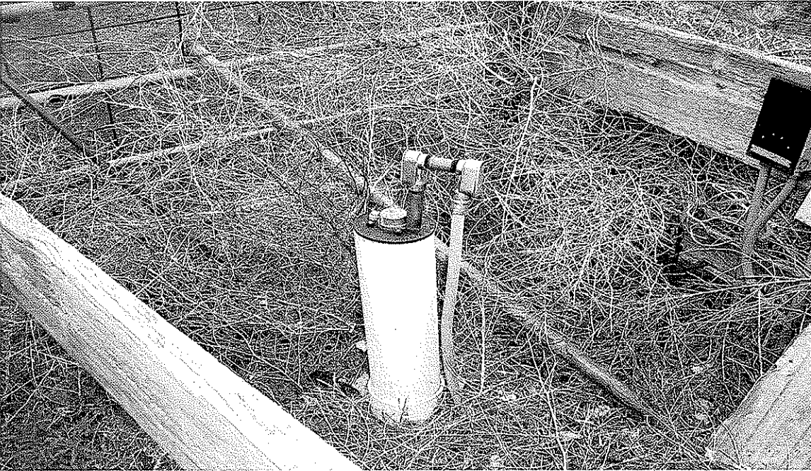
Photo 13A: Well head.
