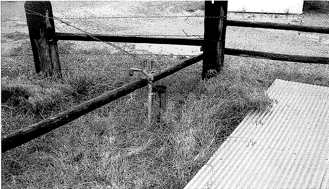
Photo 15B: Sample spigot looking west, next to well vault.
