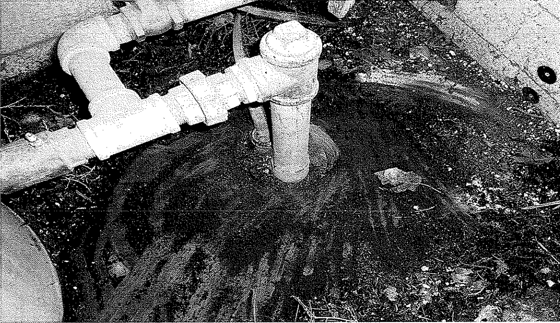
Photo 19A: Well head in small shed.
