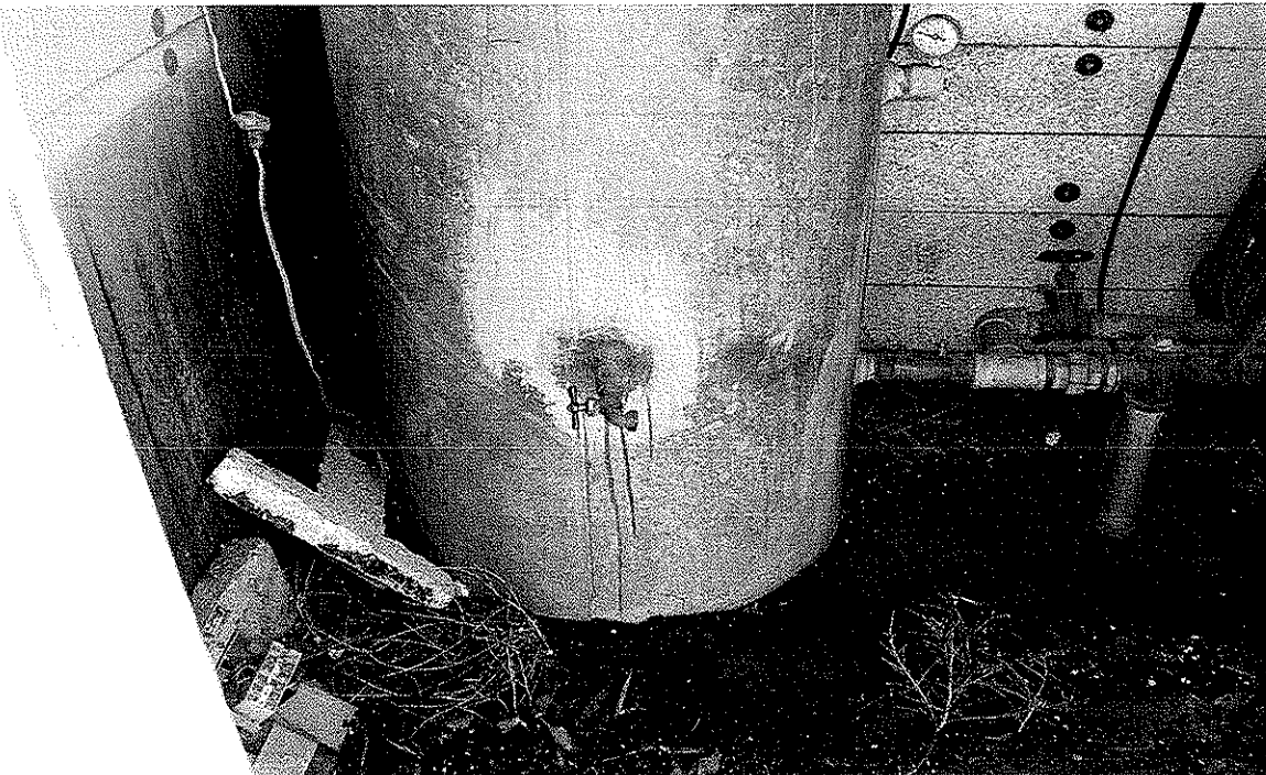
Photo 19B: Sample spigot out of pressure tank next to well head.
