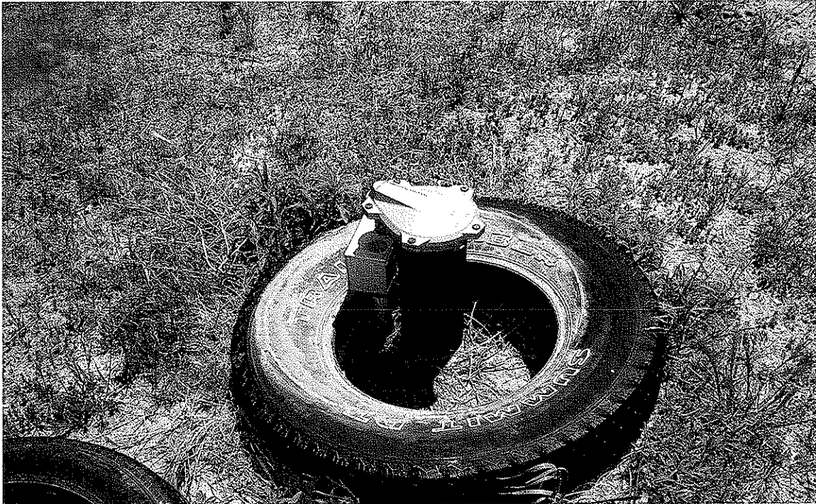
Photo 24A: Well head.
