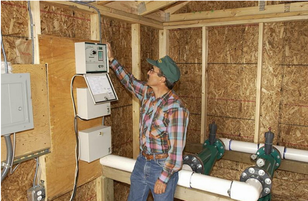
Figure 7. View of the filtration system and control panel.
