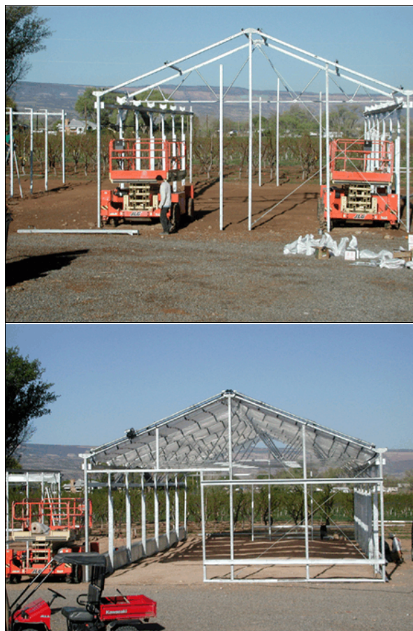
Fig. 4. A progression of construction of two retractable roof greenhouses at Western Colorado Research Center – Orchard Mesa during spring 2002. (photos by Harold Larsen)
