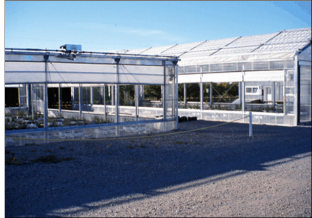
Fig. 6. A view of partially constructed and completed greenhouses – the side walls are open, the roof covering is closed. (Photo by Matt Rogowski).
