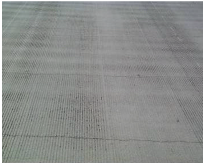
Figure F.3 Crack pattern at the mid-span (3.5 ft spacing)
