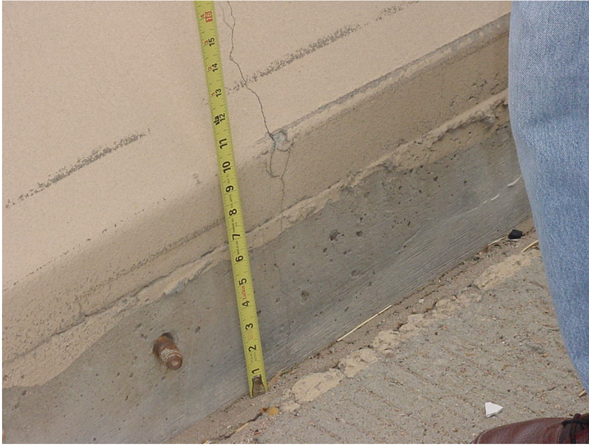
Figure C.5. A Settlement of 6” Between the Roadway and the Bridge Concrete Rail: North-East Side of Structure E-17-SW in Region 6.
