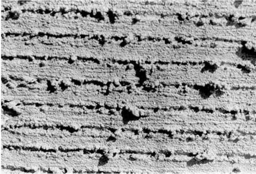
Photo 4: Popcorn-like mortar balls (longitudinal tining)
