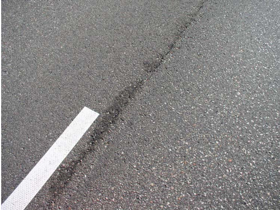
Figure 12. Early Deterioration of Longitudinal Joint, Note Moisture in Joint (2003)
