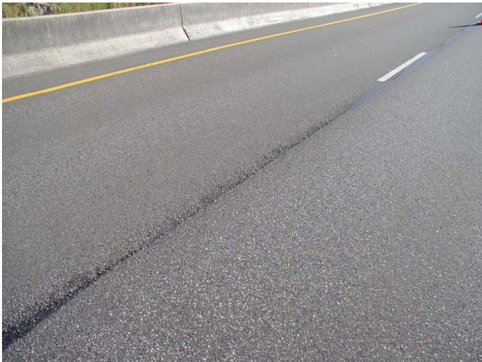
Figure 13. Raveling at Longitudinal Joint
