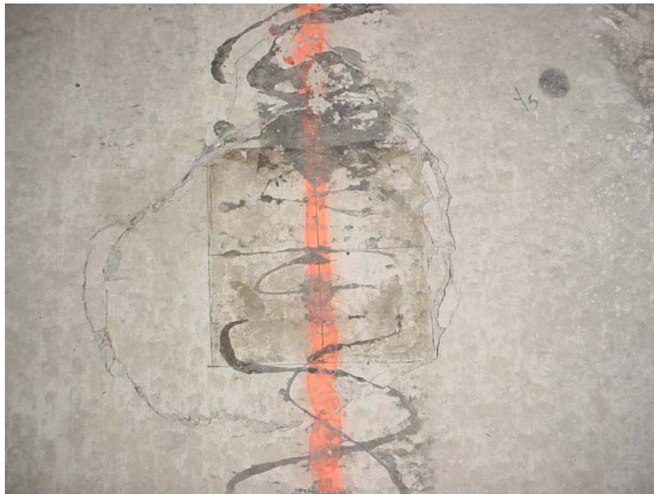
Figure 6.23 – Punching Shear Crack
