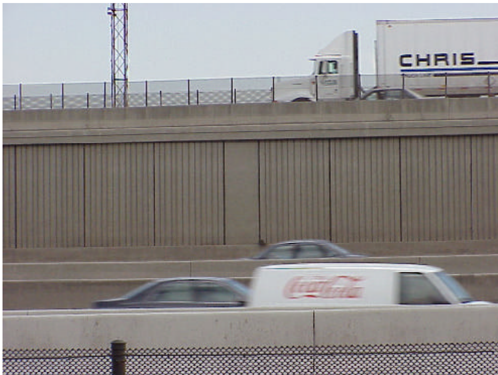
This mechanically stabilized earth wall, with independent full-height facing, is part of the ramp connecting N.B. I25 to I70 in Denver.
