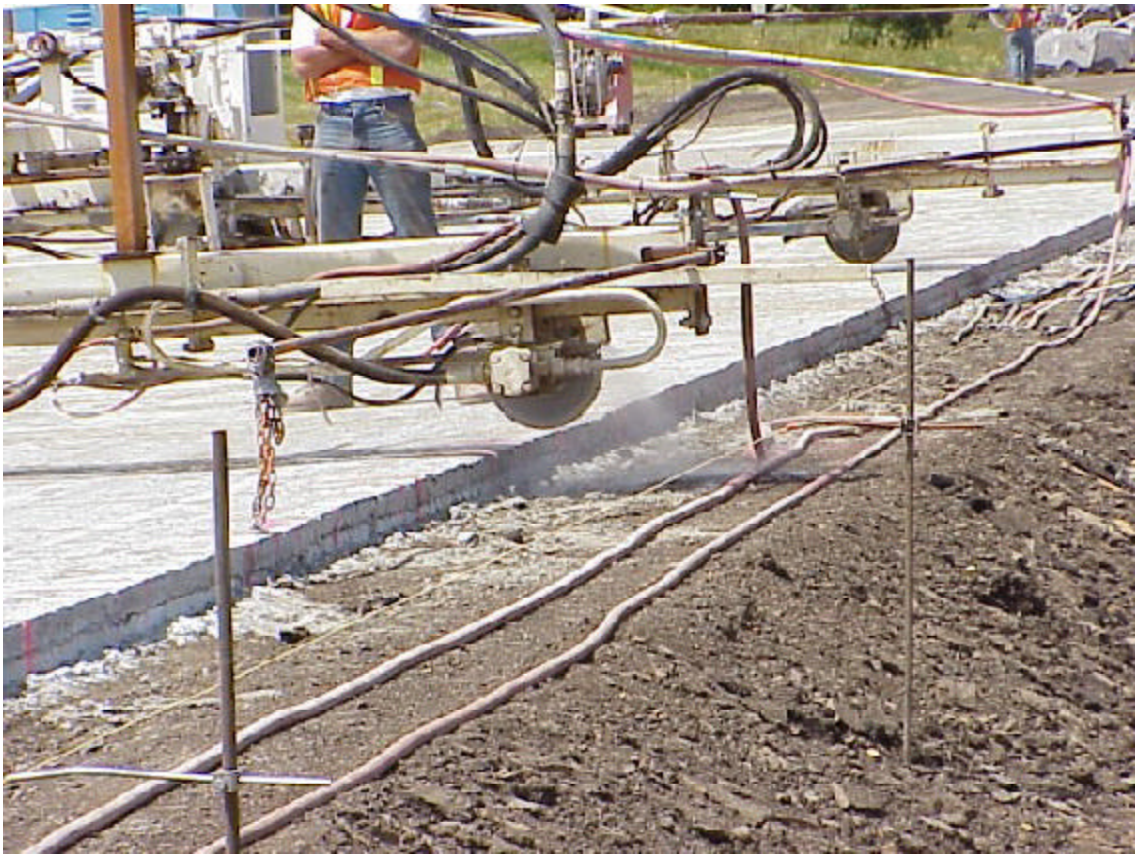
Whitetopping is a thin concrete overlay over asphalt pavement. It is used as a rehabilitation method.
