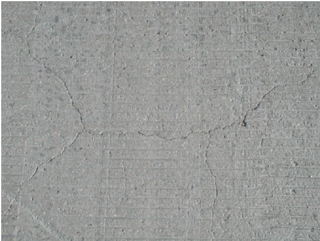
This bridge deck is showing extensive cracking.
