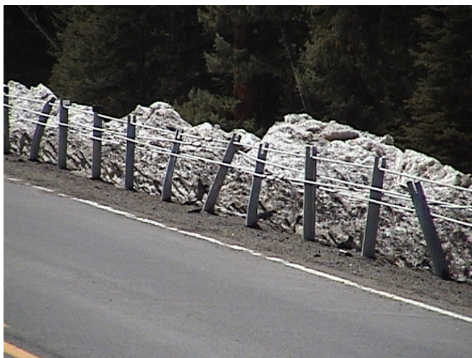
Figure 5. Posts on SH-65 are bent in all directions, suggesting that the damage is not all caused by snowplows.
