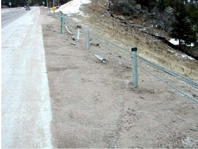
Figure 1. The most severe hit on the Windy Point systems damaged only six posts.
