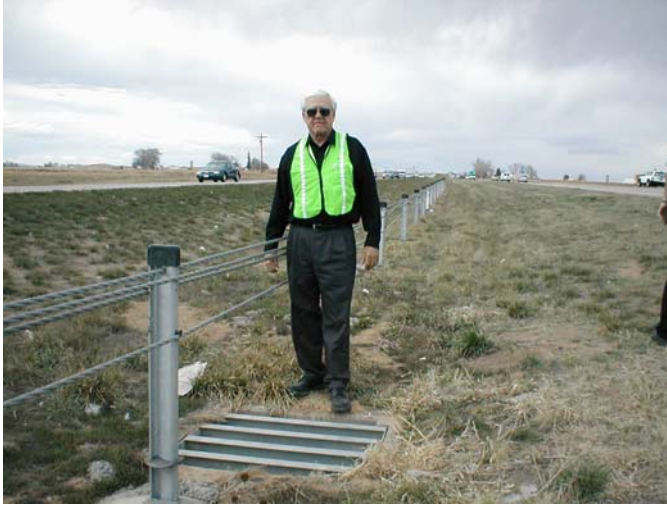
Figure 4. The cables over this drain inlet are much farther off the ground than the design specification.
