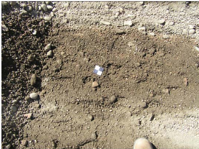
Figure 4. Mt. Vernon Canyon's 1/2" pea gravel arrester bed is heavily polluted by fine material. A quantity of 1" aggregate was added to the bed at some time.
