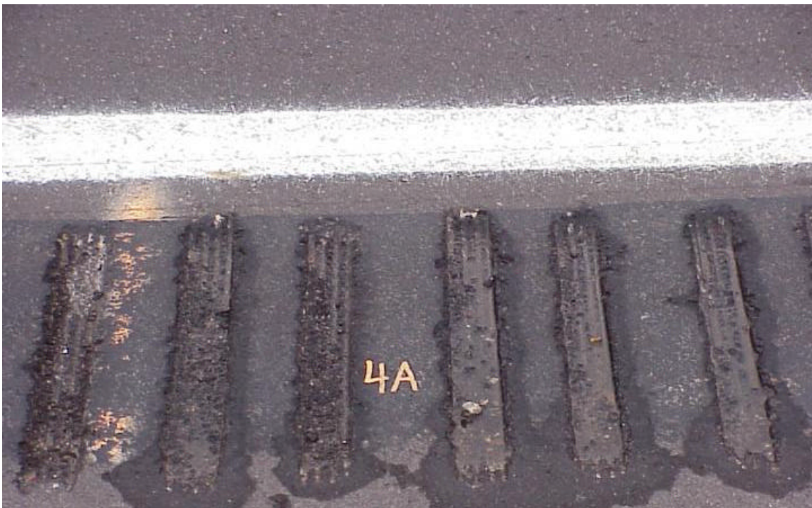
Figure 14. Test section 4A on I 70 at Eagle - 2" groove 3" flat. This picture shows how the rumble strip may capture water and debris. The slight variations in the groove spacing are caused by the spacers used on the grinding drum.
