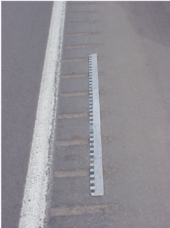
Figure A-1. At Eagle on I 70 eastbound , CDOT constructed nine rumble strip configurations. This figure shows the spacing of the grooves in section 1 – the first section at the west end of the test sections. The black and white squares on the straight edge are one inch on a side. The straight edge shows that the grooves are 2” wide with 10” flats in between. This spacing was ground for 1000 feet in a continuous configuration and then for another 1000 feet in an interrupted configuration – 12 feet of grooves and 6 feet without grooves.
