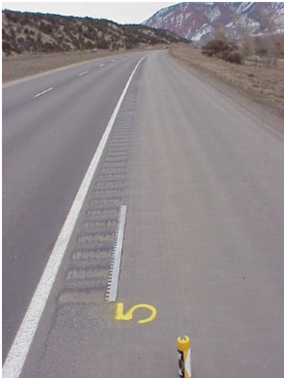
Figure A-14. Section 5 was ground in an interrupted pattern. The old standard style rumble strip has 12 foot gaps after 48 feet of rumble strip. The white arrow points to a gap in the rumble strip.
