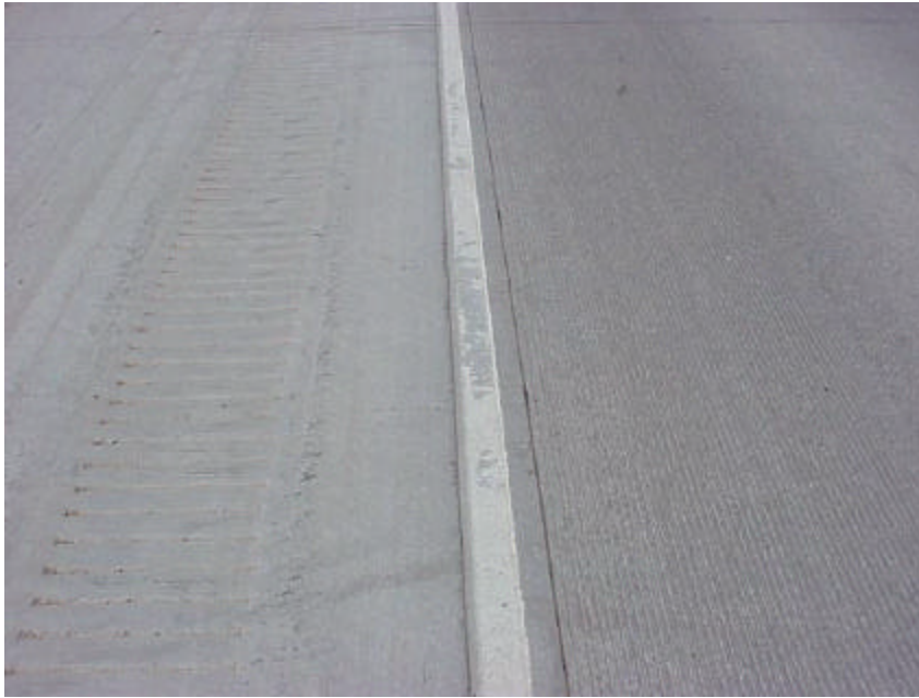
Figure A-19. The concrete rolled-in rumble strip used for the study was placed away from the shoulder stripe at the request of CDOT maintenance.
