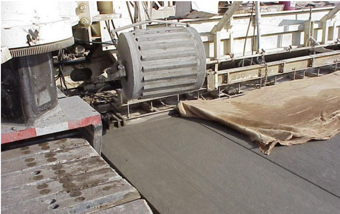
Figure 15. The roller that forms rumble strips in new concrete pavement. The roller has been raised because the paving operation is approaching an intersection. This roller forms rumble strips on the left shoulder.
