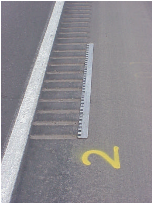
Figure A-6. Section 2 uses 2-inch grooves with 5-inch flats between. This section is continuous rumble strip.
