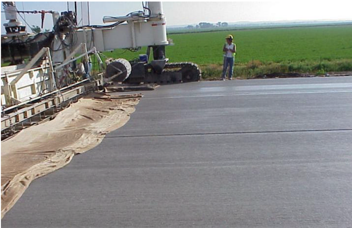
Figure 16. The roller that forms rumble strips in new concrete pavement. The roller that forms the right shoulder rumble strip can be seen at the far side of the paving machine. It has been raised off the surface because the paving operation is approaching an intersection.
