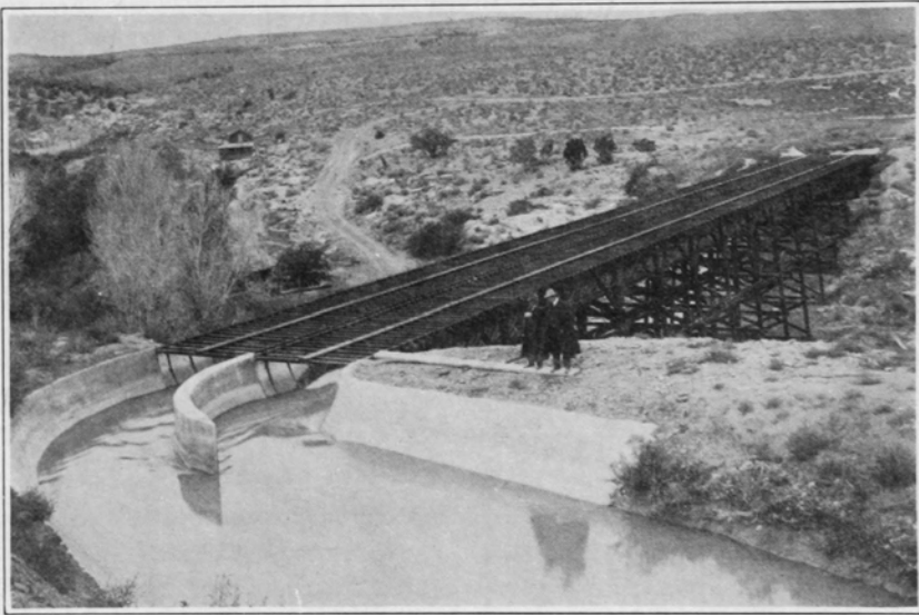
Concrete approach to the Happy Canon flume, Montrose and Delta canal, on the Uncompahgre Project
