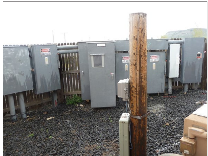
FIGURE 8: POWER DISTRIBUTION CENTER
