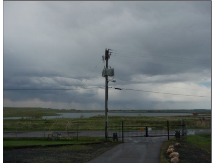
FIGURE 7: UTILITY TRANSFORMER BANK
