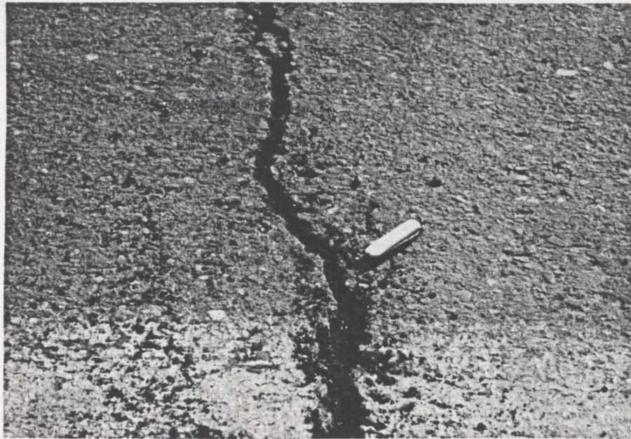
The cracks in the Gilsonite section are much wider than the cracks in the control section. August 1991 Gilsonite section
