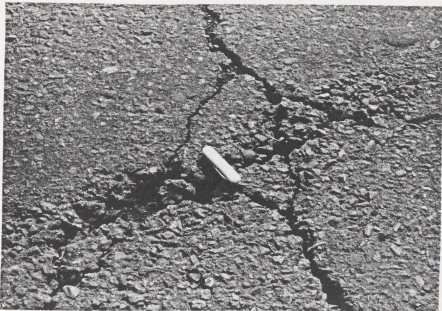
The cracks in the Gilsonite section are also deteriorating faster.
