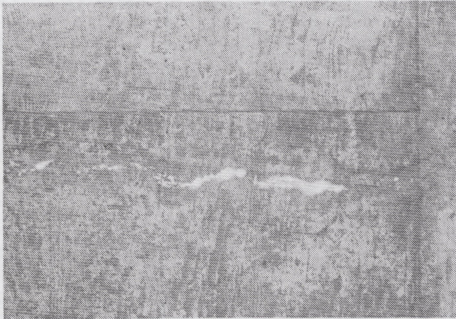
Photograph 3. Slight efflores- cence on underside of deck. Ken Caryl Rd.
