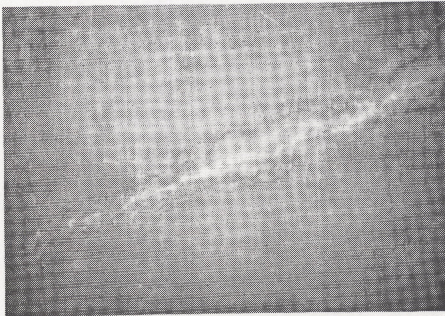
Photograph 5. Mild efflorescence on underside of deck. Kipling St.
