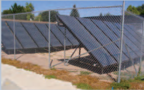
As one of many energy-efficient upgrades in Eaton School District's Performance Contracting project, Eaton High School now uses a solar hot water system to heat its swimming pool water. Photo: Eaton School District RE-2.
