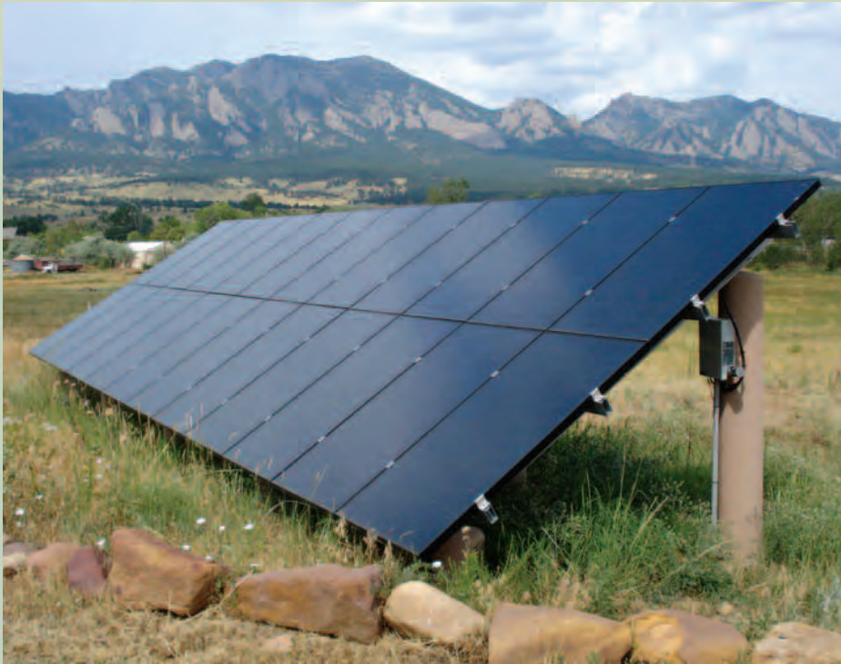
Residential ground-mount PV system, South Boulder. Photo: Simple Solar.
