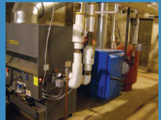
After: New, more efficient boiler system heats the room, while a solar hot water system heats the swimming pool water. Photo: Eaton School District RE-2.
