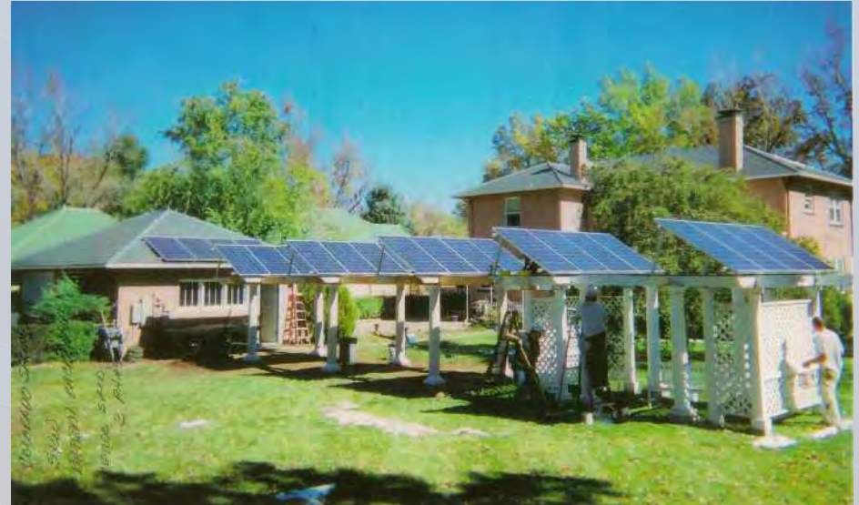
To retrofit this 1890s Colorado Springs home for solar energy, the installer was able to satisfy the Colorado Springs Utility, the Historical Society and the Colorado Springs Building Department by placing solar panels on the pergola-type arbor in the back yard. Photo: Thames Solar Electric.
