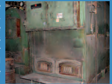
Old coal-burning boiler to be replaced at Oak Creek Middle School.
