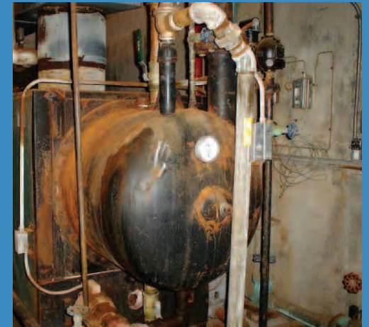
Before: This old, inefficient boiler was used year-round to heat both the swimming pool water and the swimming pool room at Eaton High School. Photo: Eaton School District RE-2.
