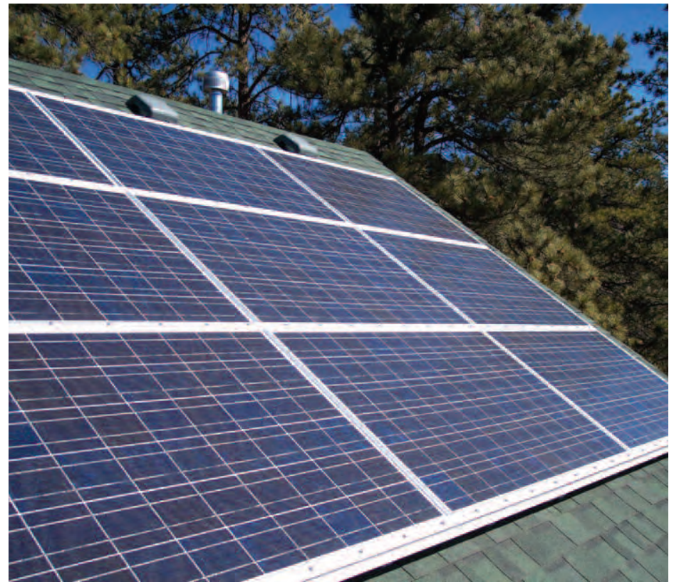
Rooftop array in Boulder County. Photo: Sun Volt Solar Electric.
