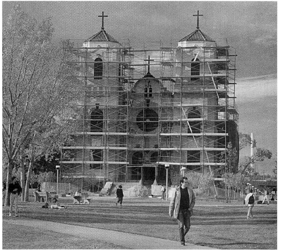
Complete exterior restoration of St. Cajetan's in 1991 included a return to its original colors. Photo by Michael Gamer
