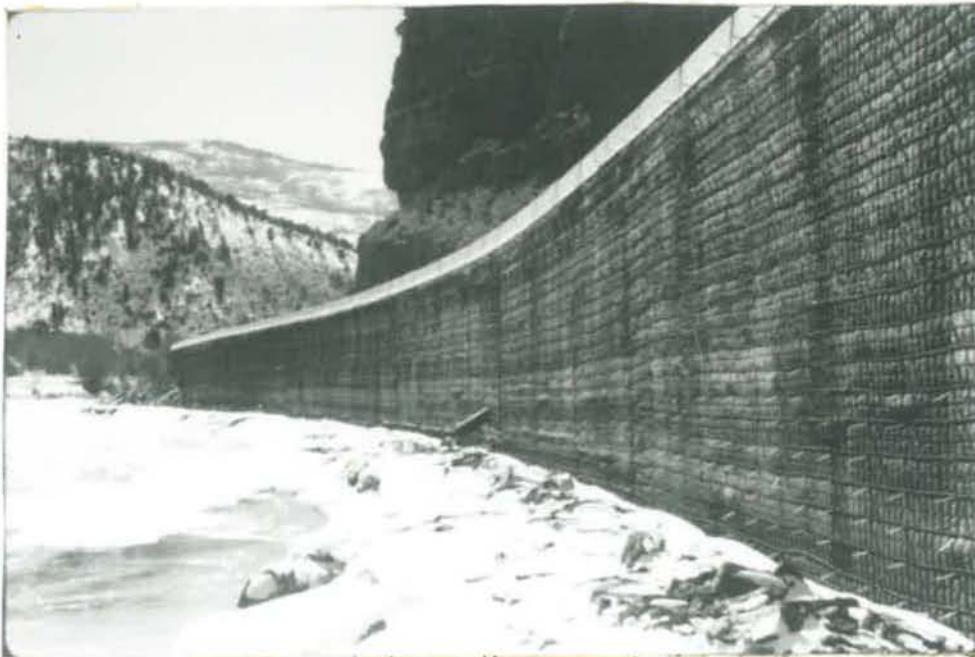
FIGURE 8 - COMPLETED WALL AT THE END OF PHASE ONE CONSTRUCTION. THE TEMPORARY FACING IS CLEARLY ILLUSTRATED.
