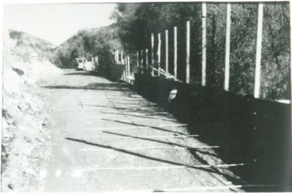
FIGURE 4 - PLACING A LAYER OF REINFORCEMENT STRIPS AND CONNECTING THEM TO THE TEMPORARY FACING
