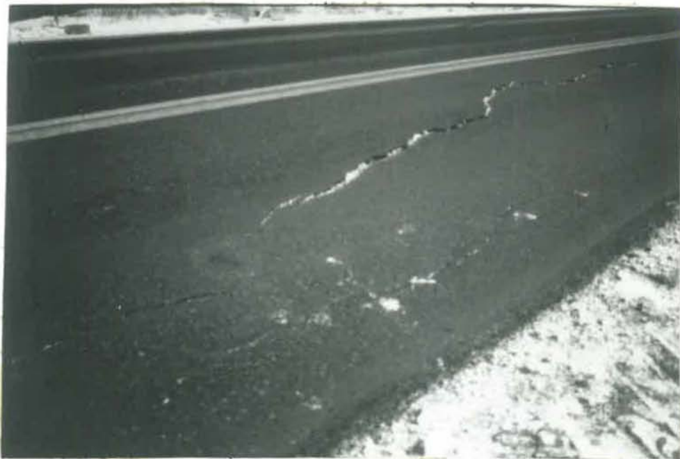
FIGURE 14 - PAVEMENT LONGITUDINAL CRACKS ON TOP OF THE TWO PHASE WALLS
