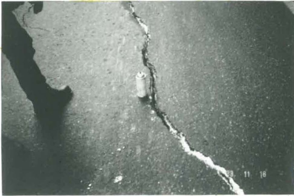
FIGURE 13 - CLOSE UP VIEW OF THE PAVEMENT CRACKS
