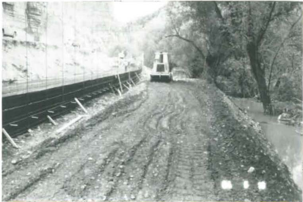
FIGURE 7 - COMPACTING THE SOIL PLACED IN FRONT OF THE REINFORCED EARTH WALL TO PROVIDE STABILITY AND THE NECESSARY AREA FOR THE FUTURE BIKE-PATH PLATFORM.
