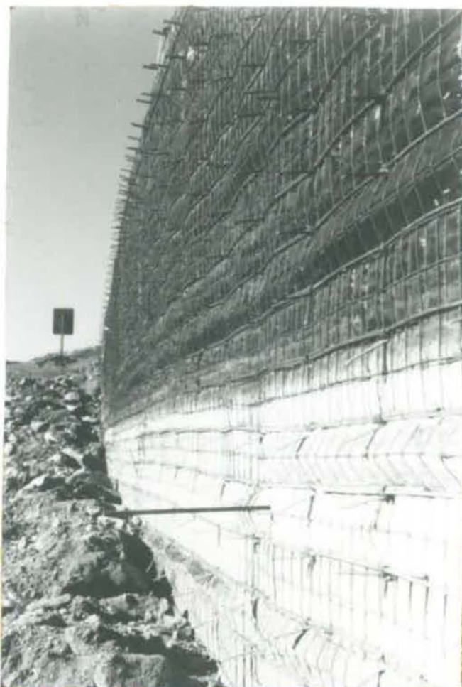
FIGURE 9 - REBARS STICKING OUT OF THE REINFORCED EARTH WALLS WERE USED AS SURVEY STATIONS
