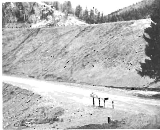
Mid June before seeding and spraying No plant growth and no erosion protection
