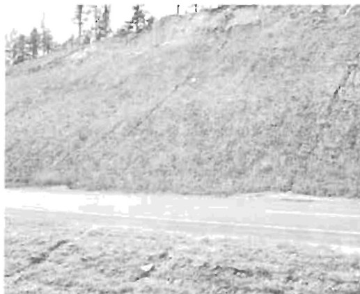
October About 40% Plant Cover Gullies Appearing in Slope
