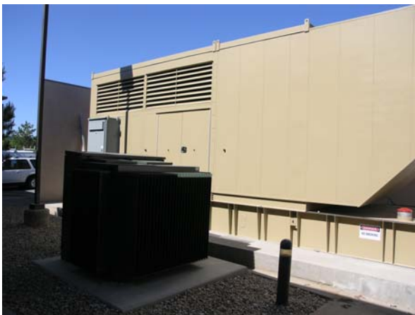
e-FOR 3T 's - 2 Mega Watt Emergency Generator
