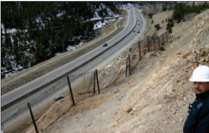
Figure 11: Wire rope rockfall fence installed on a rock slope at Georgetown Hill above Interstate 70. Exit ramps shown in the upper part of the photo are for the Silver Plume Exit. (Photo courtesy of Ty Ortiz, CDOT.)
