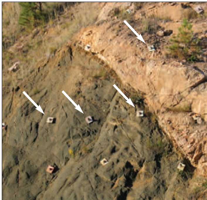
Figure 13: Pattern rock bolting to reinforce the rock cut along Highway 285. The threaded steel bars have been cemented into drill holes. The external evidence of rock reinforcement is shown by the steel plates and large nuts, four of which are indicated with arrows. (Photo by TC Wait.)
