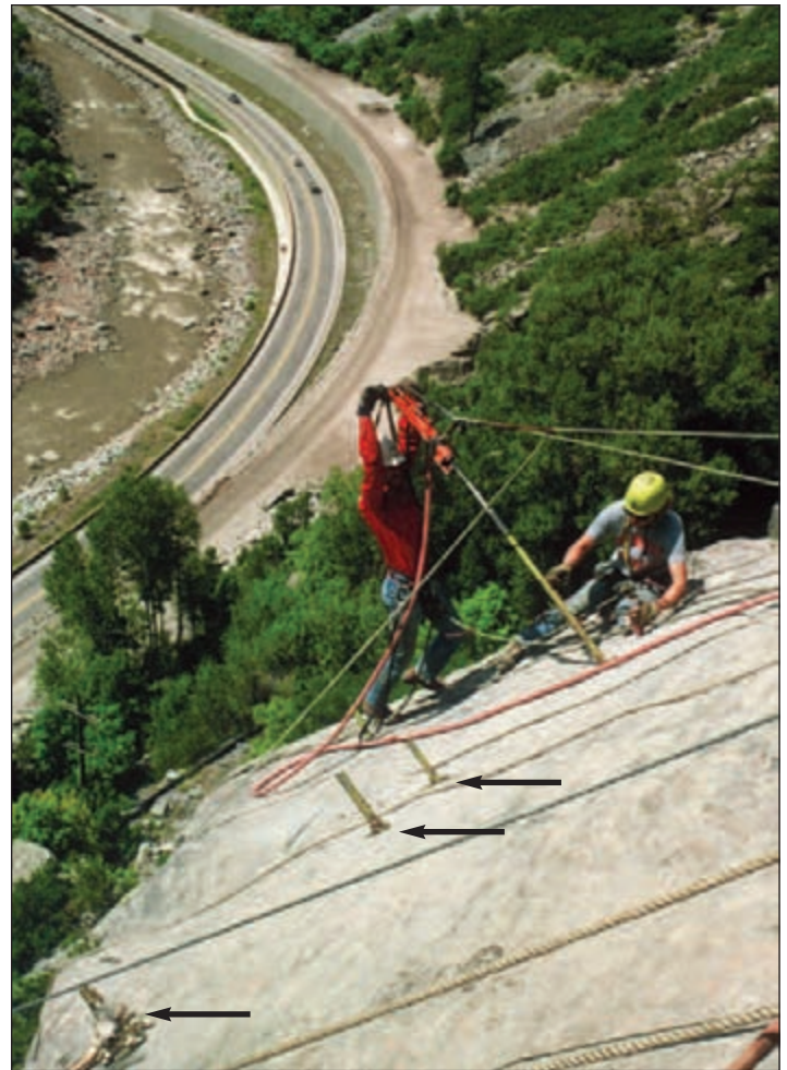
Figure 12: Installation of rockbolts on the rocky slope of Glenwood Canyon during the Interstate 70 highway construction project in 1991. The worker is spinning an epoxy-coated steel bar into the drill hole using a pneumatic drill. The protruding bars in the foreground (shown by arrows) are installed rockbolts. (Photo by Jon White.)
