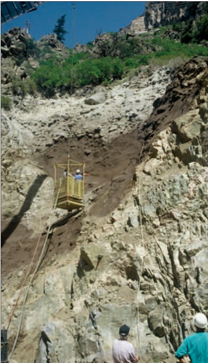
Figure 15: Application of shotcrete at a raveling cut-slope exposed in a rocky talus chute. The concrete has been dyed dark brown to better match the surrounding area. (Photo by Jon White.)
