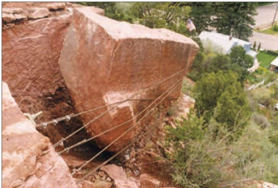
Figure H: A precarious rock above Manitou Springs started to move in 1995 after a period of wet weather. As an emergency measure, high-strength steel cables were wrapped around the rock and anchored to the surrounding ledge to arrest the movement. (Photo by Jon White.)
