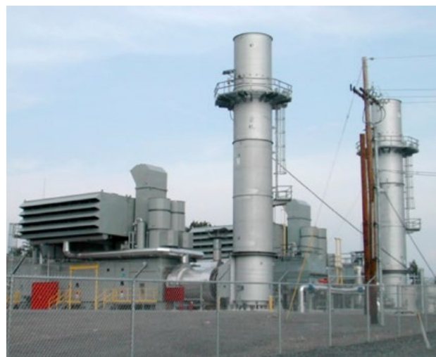
FIGURE 1-9: 44 MW GAS TURBINES AT VP#8 AND BUCHANAN PROJECT (SOURCE: CONSOL ENERGY)
