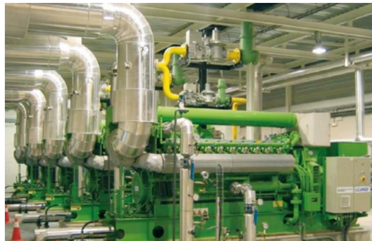
FIGURE 1-4: GE JENBACHER IC ENGINES USING CMM (SOURCE: GENERAL ELECTRIC)
