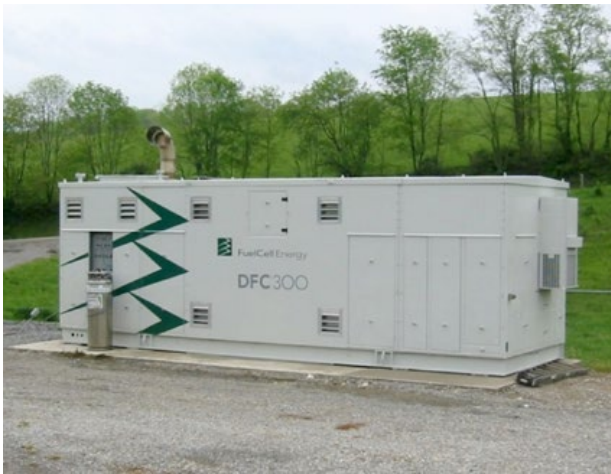
FIGURE 1-12: 200KW FUEL CELL AT ROSE VALLEY MINE (SOURCE: U.S. EPA)
